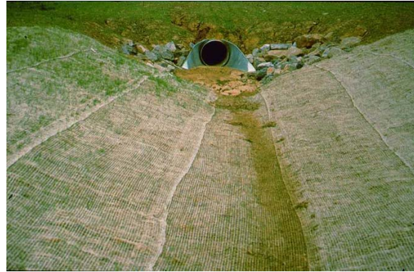
5-16 Good netting installation, but problems at pipe outlet need to be addressed.
