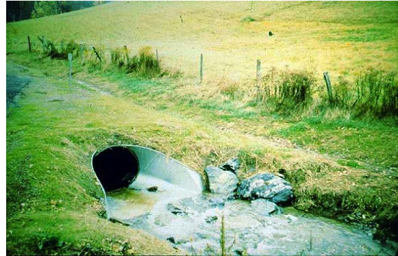
5-36 Metal flared end section on plastic pipe.
