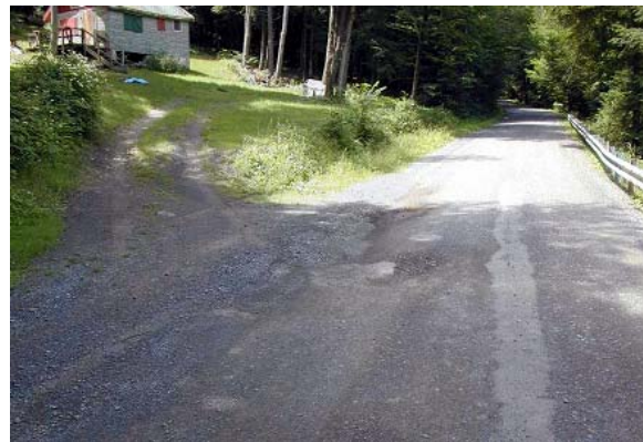
ESMP#6-01 Improperly constructed driveways not only cause road drainage and road safety hazards, but also cause degradation of the environment through erosion and sediment.
