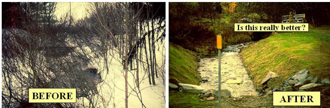
6-17 Clearing stream banks for a road crosspipe replacement can have devastating effects on the stream and future maintenance.
