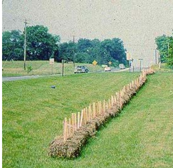
5-04 Proper bale installation prior to start of a major construction project. (Note: Bale barriers not recommended by EPA.)
