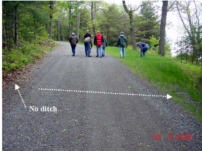
ESMP#2-01 Outsloped road showing no ditches and vegetative filtering areas for overland sheet flows.
