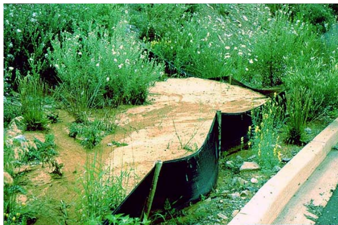
5-07 Cleaning is required when sediment reaches one-half the height of the fence.
