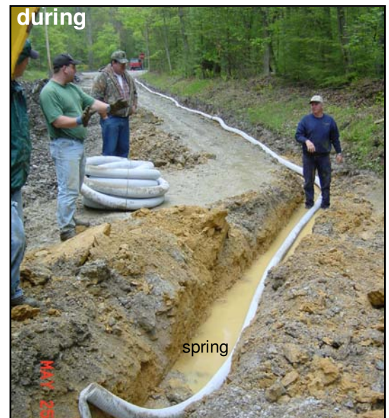
Photo 2. Pre-fabricated underdrain was used to collect subsurface water from under the road and both ditches.
