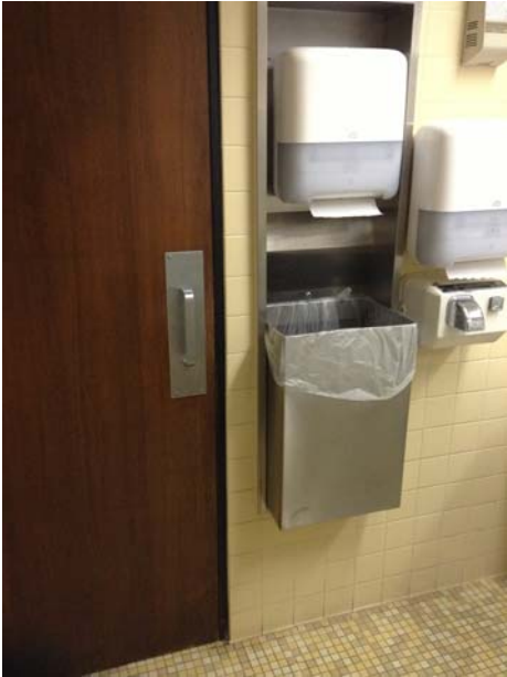
22 Restroom Violation 1D
