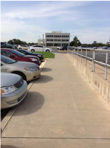
13 Accessible Route Violation 4B
