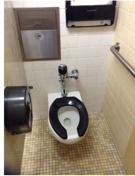
21 Restroom Violation 1C
