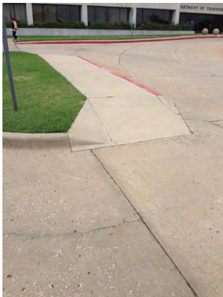
7 Accessible Route Violation 2
