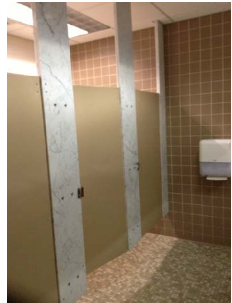
48 Restroom Violation 8B
