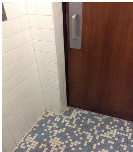
44 Restroom Violation 7B
