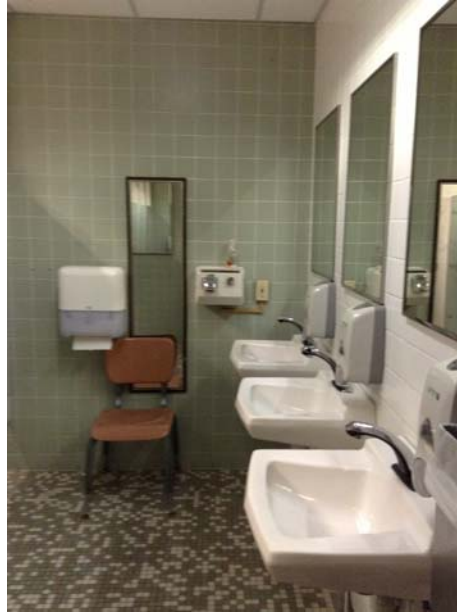
56 Restroom Violation 9G
