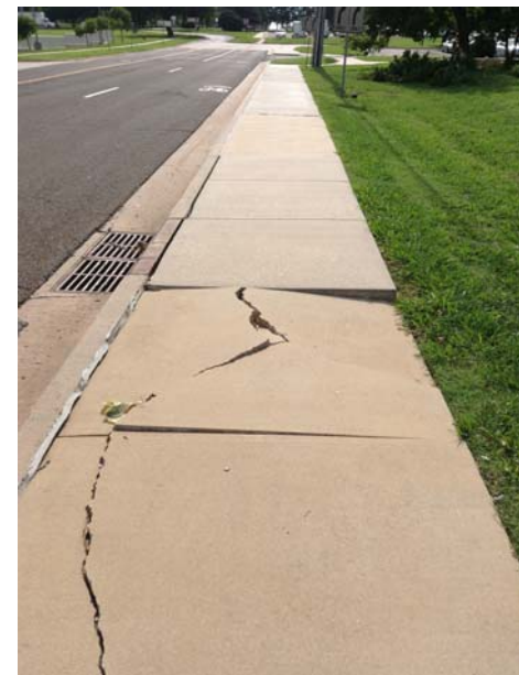
9 Accessible Route Violation 2C
