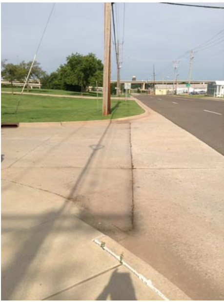
10 Accessible Route Violation 2D
