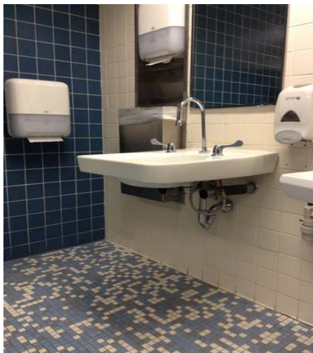
53 Restroom Violation 9D
