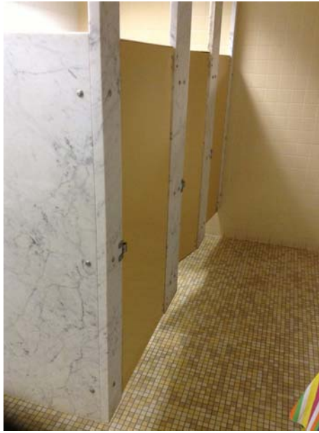
20 Restroom Violation 1B
