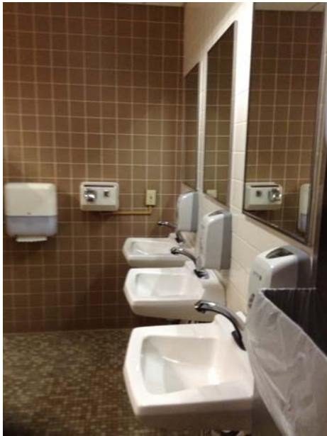
49 Restroom Violation 8C
