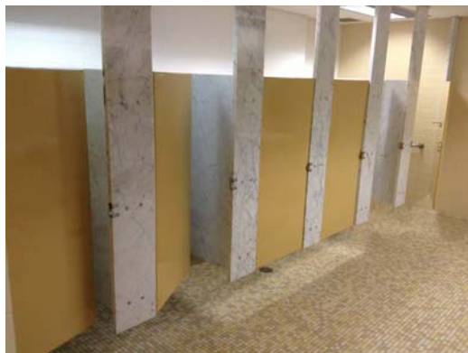
35 Restroom Violation 4C
