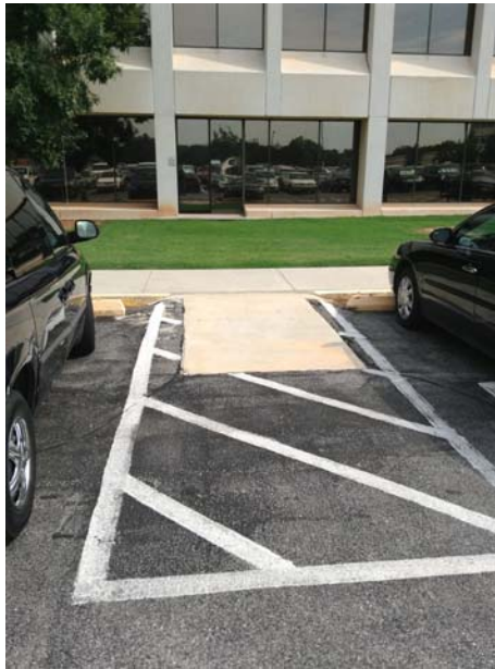
14 Accessible Route Violation 5
