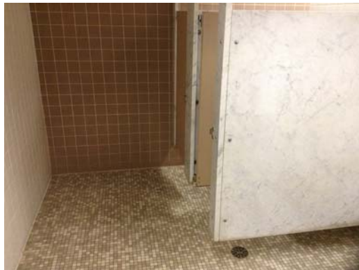
26 Restroom Violation 2D
