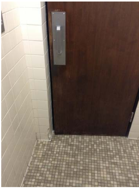
55 Restroom Violation 9F
