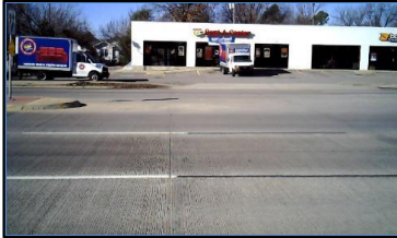
Corner 4 No Ramp (4z)
