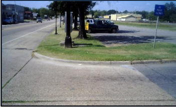
Corner 1 No Ramp (1z)
