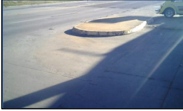
Corner 3 No Ramp (3z)
