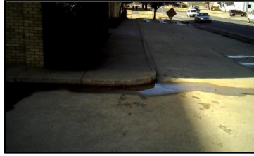
Corner 4 No Ramp (4z)
