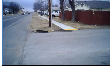
Corner 2 No Ramp (2z)
