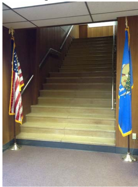
2. Accessible Route Violation 2
