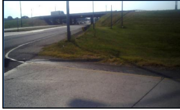
Corner 1 No Ramp (1z)
