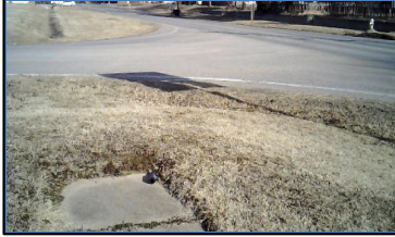
Corner 4 No Ramp (4z)
