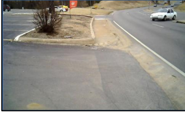
Corner 3 No Ramp (3z)
