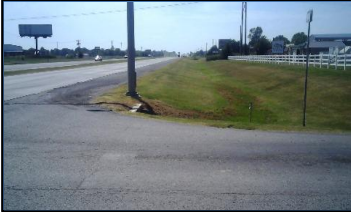
Corner 4 No Ramp (4z)
