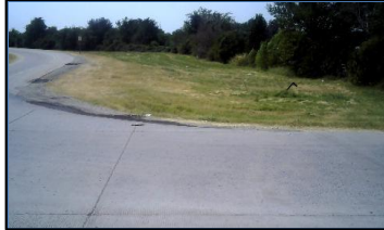
Corner 4 No Ramp (4z)
