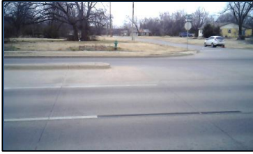
Corner 1 No Ramp (1z)
