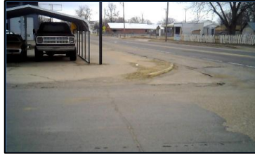
Corner 2 No Ramp (2z)
