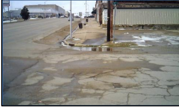
Corner 1 No Ramp (1z)
