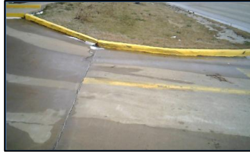
Corner 2 No Ramp (2z)
