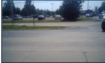
Corner 3 No Ramp (3z)
