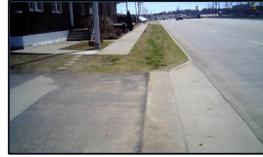
Corner 3 No Ramp (3z)
