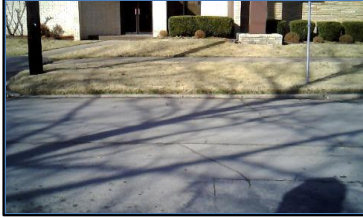
Corner 4 No Ramp (4z)
