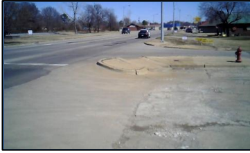
Corner 3 No Ramp (3z)
