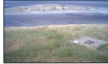
Corner 2 No Ramp (2z)
