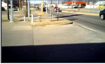
Corner 1 No Ramp (1z)
