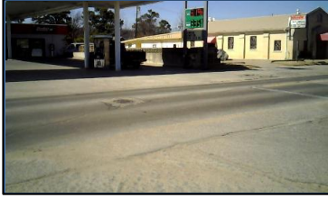
Corner 1 No Ramp (1z)
