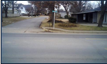
Corner 4 No Ramp (4z)
