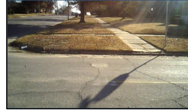
Corner 3 No Ramp (3z)
