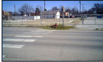
Corner 2 No Ramp (2z)
