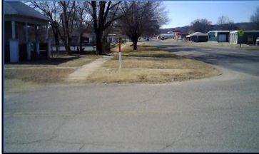
Corner 4 No Ramp (4z)
