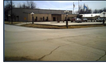
Corner 3 No Ramp (3z)
