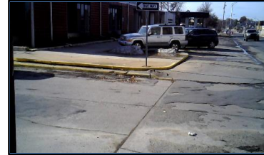
Corner 4 No Ramp (4z)
