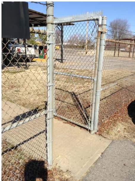
2. Accessible Route Violation 1
