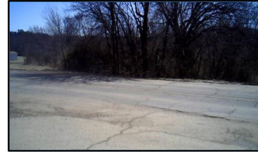
Corner 3 No Ramp (3z)
