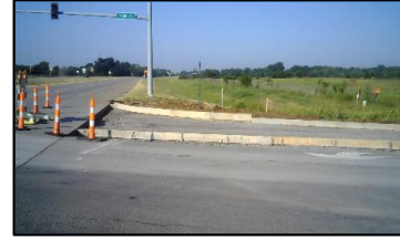
Corner 1 No Ramp (1z)
