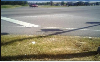
Corner 1 No Ramp (1z)
