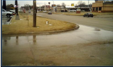
Corner 4 No Ramp (4z)
