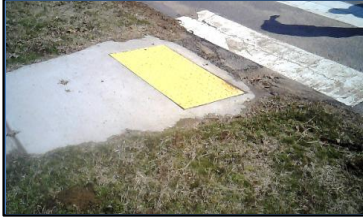
Corner 1 No Ramp (1z)
