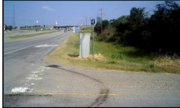
Corner 3 No Ramp (3z)
