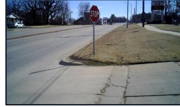
Corner 3 No Ramp (3z)
