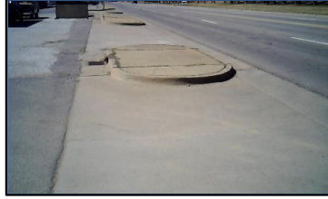
Corner 4 No Ramp (4z)
