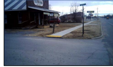
Corner 3 No Ramp (3z)
