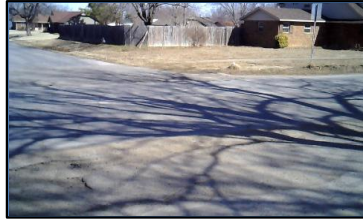
Corner 2 No Ramp (2z)
