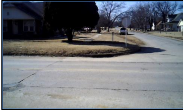
Corner 4 No Ramp (4z)
