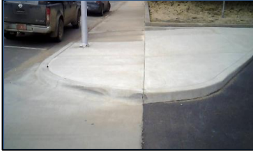
Corner 1 No Ramp (1z)
