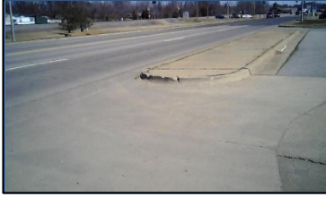
Corner 3 No Ramp (3z)
