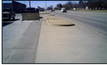
Corner 4 No Ramp (4z)
