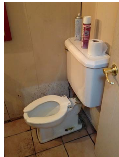
9. Restroom Violation 1C
