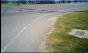
Corner 4 No Ramp (4z)
