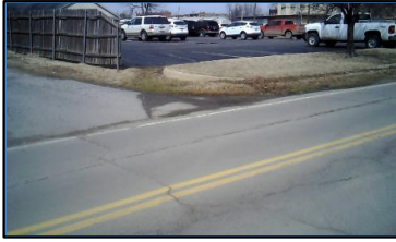
Corner 1 No Ramp (1z)
