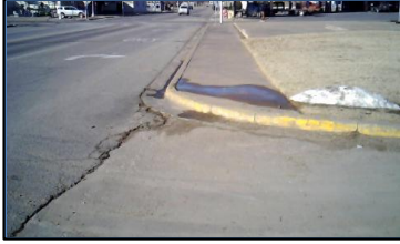
Corner 2 No Ramp (2z)
