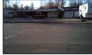
Corner 3 No Ramp (3z)
