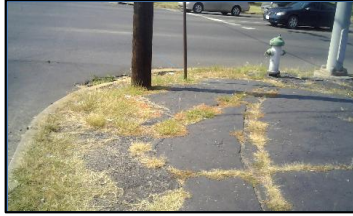
Corner 2 No Ramp (2z)
