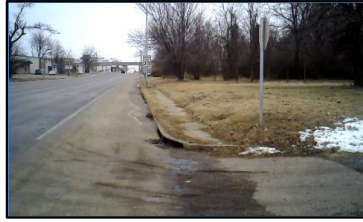
Corner 2 No Ramp (2z)
