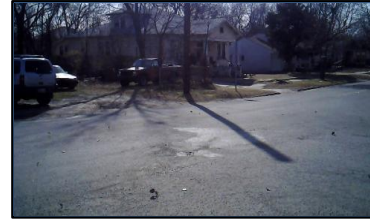
Corner 3 No Ramp (3z)
