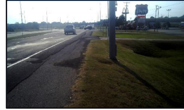
Corner 1 No Ramp (1z)
