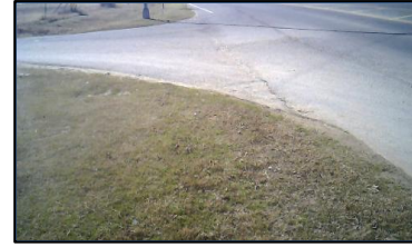
Corner 3 No Ramp (3z)
