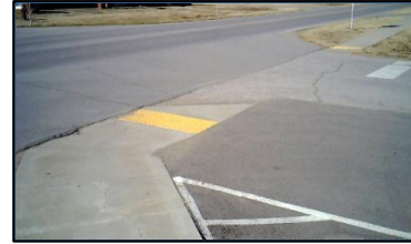
Corner 3 No Ramp (3z)
