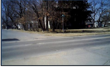
Corner 1 No Ramp (1z)
