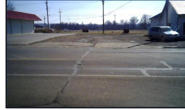
Corner 3 No Ramp (3z)
