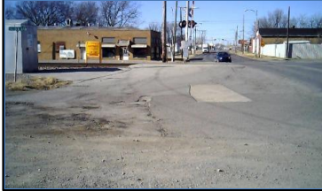
Corner 4 No Ramp (4z)
