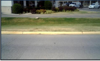
Corner 1 No Ramp (1z)
