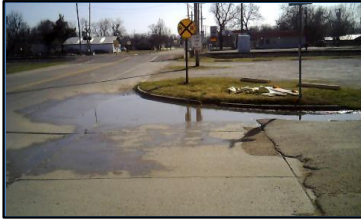
Corner 1 No Ramp (1z)
