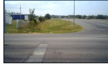
Corner 3 No Ramp (3z)
