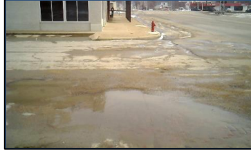
Corner 2 No Ramp (2z)
