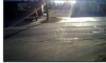
Corner 3 No Ramp (3z)
