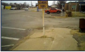
Corner 1 No Ramp (1z)
