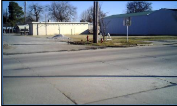
Corner 4 No Ramp (4z)
