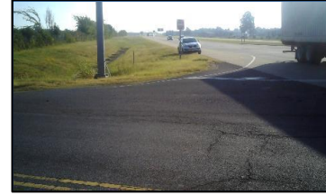
Corner 2 No Ramp (2z)
