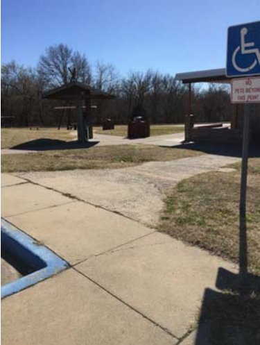
3. Accessible Route Violation 1
