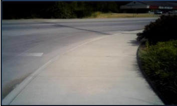
Corner 4 No Ramp (4z)
