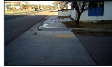
Corner 3 No Ramp (3z)
