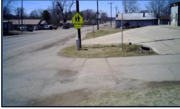
Corner 1 No Ramp (1z)
