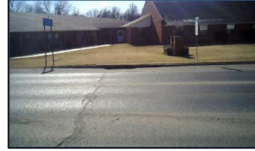
Corner 3 No Ramp (3z)
