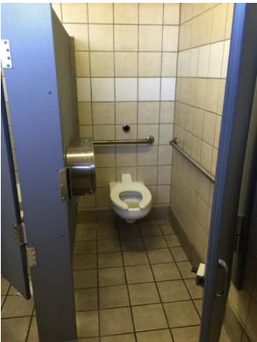
9. Restroom Violation 1C
