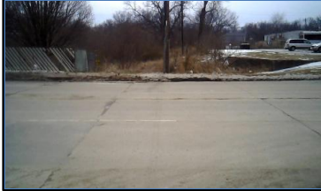
Corner 4 No Ramp (4z)
