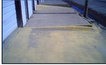
Corner 2 No Ramp (2z)
