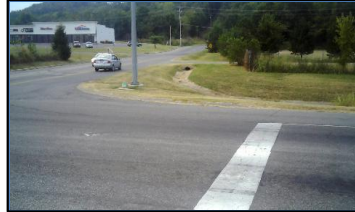
Corner 4 No Ramp (4z)
