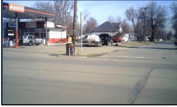
Corner 1 No Ramp (1z)
