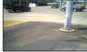
Corner 3 No Ramp (3z)
