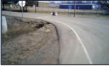
Corner 1 No Ramp (1z)
