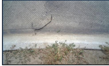
Corner 2 No Ramp (2z)
