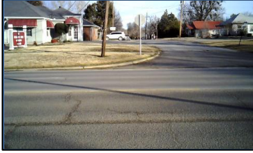
Corner 1 No Ramp (1z)
