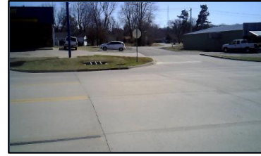
Corner 3 No Ramp (3z)
