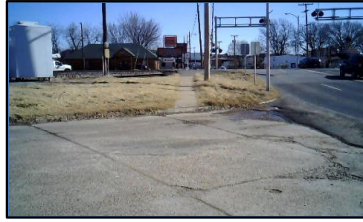
Corner 2 No Ramp (2z)
