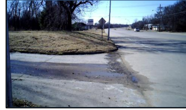
Corner 3 No Ramp (3z)
