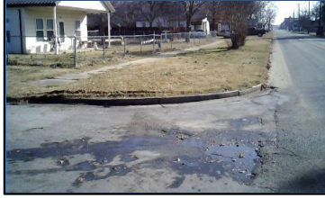
Corner 2 No Ramp (2z)
