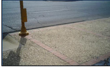
Corner 2 No Ramp (2z)
