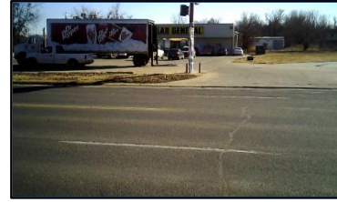
Corner 3 No Ramp (3z)
