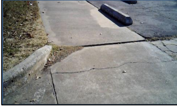
Corner 3 No Ramp (3z)
