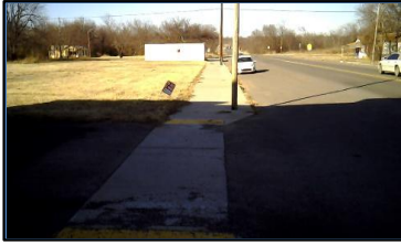
Corner 1 No Ramp (1z)
