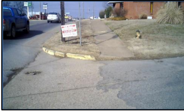
Corner 1 No Ramp (1z)
