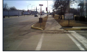
Corner 3 No Ramp (3z)
