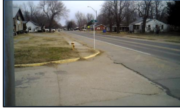
Corner 2 No Ramp (2z)
