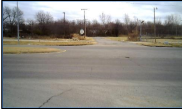
Corner 2 No Ramp (2z)
