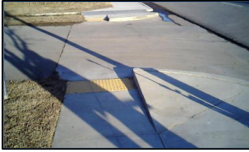
Corner 1 No Ramp (1z)
