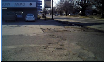
Corner 4 No Ramp (4z)
