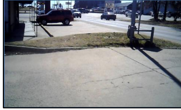
Corner 3 No Ramp (3z)
