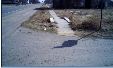
Corner 4 No Ramp (4z)
