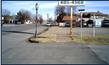
Corner 3 No Ramp (3z)
