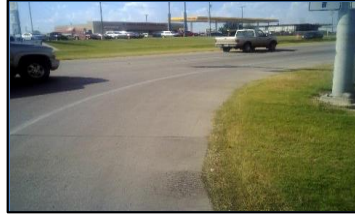
Corner 2 No Ramp (2z)
