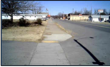
Corner 1 No Ramp (1z)
