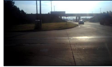
Corner 2 No Ramp (2z)
