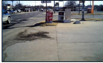
Corner 4 No Ramp (4z)
