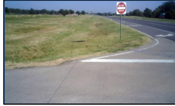
Corner 1 No Ramp (1z)
