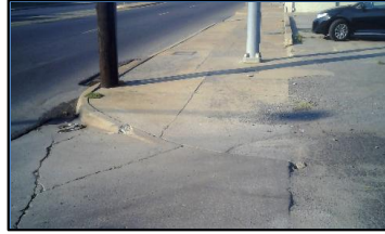
Corner 2 No Ramp (2z)
