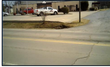
Corner 2 No Ramp (2z)
