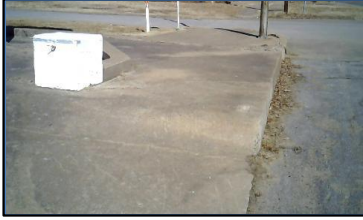
Corner 1 No Ramp (1z)
