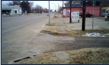
Corner 4 No Ramp (4z)
