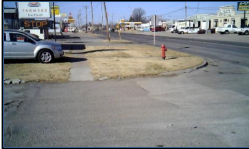
Corner 4 No Ramp (4z)
