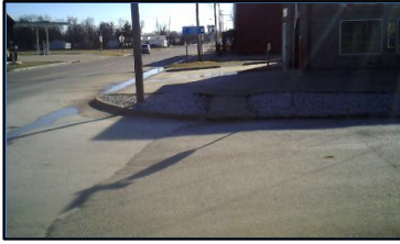
Corner 1 No Ramp (1z)
