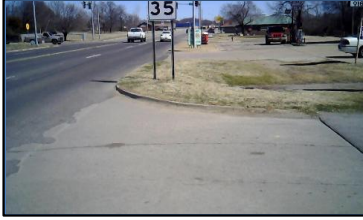
Corner 3 No Ramp (3z)
