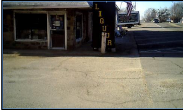
Corner 3 No Ramp (3z)
