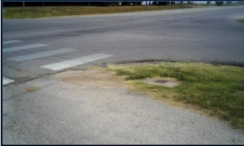
Corner 4 No Ramp (4z)
