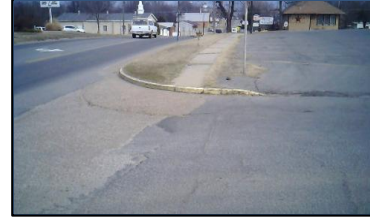
Corner 3 No Ramp (3z)
