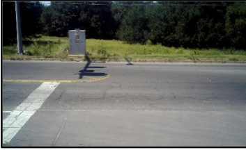
Corner 1 No Ramp (1z)
