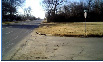
Corner 1 No Ramp (1z)
