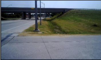
Corner 3 No Ramp (3z)
