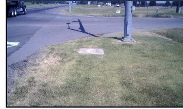
Corner 3 No Ramp (3z)
