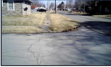
Corner 1 No Ramp (1z)
