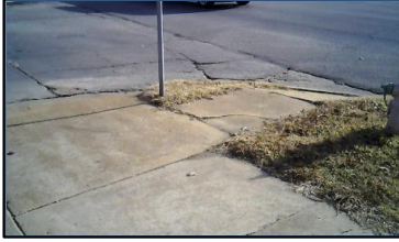
Corner 1 No Ramp (1z)
