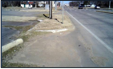
Corner 1 No Ramp (1z)
