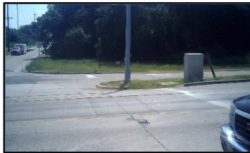
Corner 4 No Ramp (4z)
