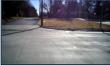
Corner 4 No Ramp (4z)
