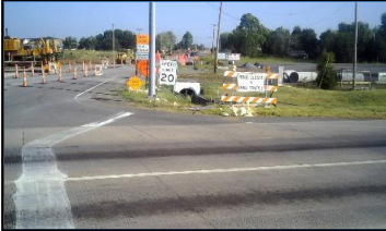
Corner 2 No Ramp (2z)
