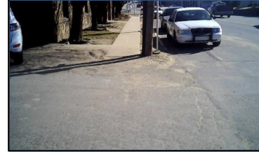
Corner 3 No Ramp (3z)
