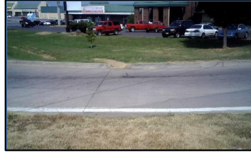
Corner 1 No Ramp (1z)
