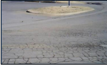
Corner 1 No Ramp (1z)
