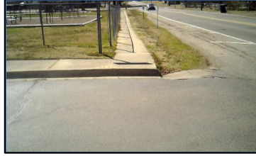
Corner 3 No Ramp (3z)
