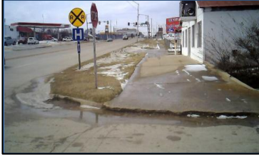
Corner 1 No Ramp (1z)
