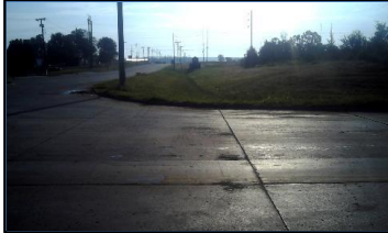
Corner 3 No Ramp (3z)
