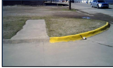
Corner 4 No Ramp (4z)
