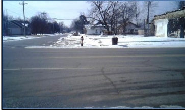
Corner 4 No Ramp (4z)
