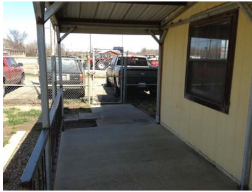
2. Accessible Route Violation 1
