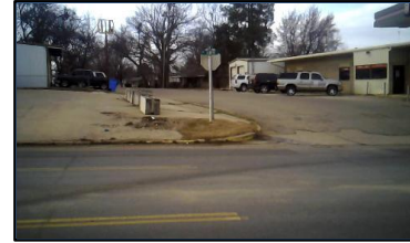
Corner 3 No Ramp (3z)
