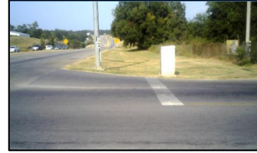
Corner 1 No Ramp (1z)
