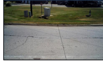
Corner 3 No Ramp (3z)
