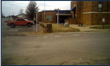
Corner 4 No Ramp (4z)
