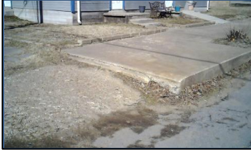
Corner 1 No Ramp (1z)
