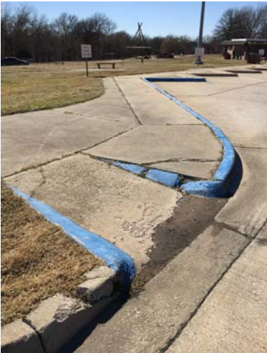
6. Accessible Route Violation 1D
