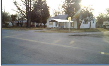
Corner 4 No Ramp (4z)
