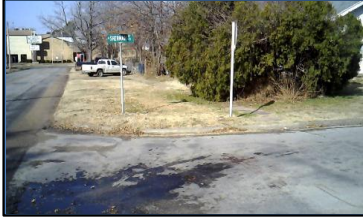
Corner 1 No Ramp (1z)
