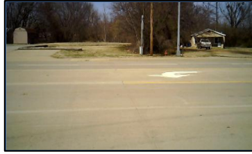
Corner 2 No Ramp (2z)
