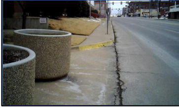
Corner 1 No Ramp (1z)
