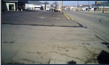
Corner 4 No Ramp (4z)
