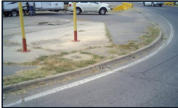
Corner 4 No Ramp (4z)
