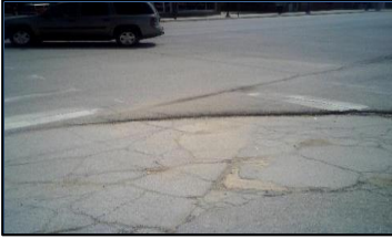
Corner 1 No Ramp (1z)
