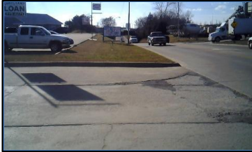
Corner 4 No Ramp (4z)
