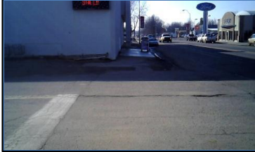
Corner 4 No Ramp (4z)
