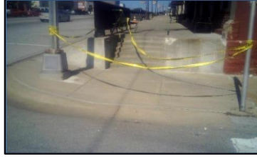
Corner 2 No Ramp (2z)
