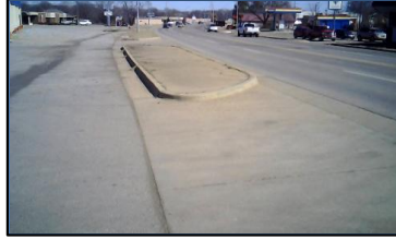
Corner 2 No Ramp (2z)
