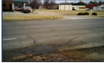
Corner 2 No Ramp (2z)
