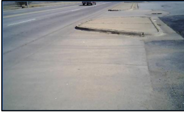
Corner 3 No Ramp (3z)
