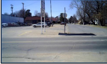
Corner 4 No Ramp (4z)
