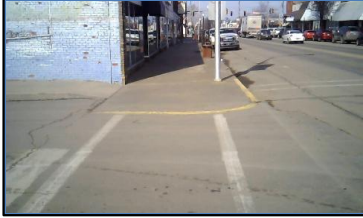
Corner 4 No Ramp (4z)
