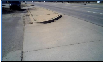
Corner 4 No Ramp (4z)
