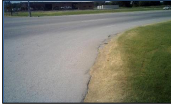
Corner 2 No Ramp (2z)
