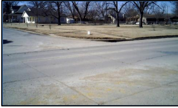
Corner 1 No Ramp (1z)
