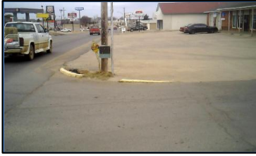
Corner 1 No Ramp (1z)
