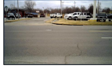
Corner 3 No Ramp (3z)
