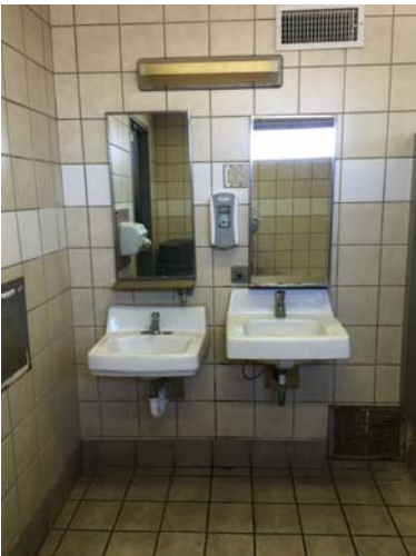
8. Restroom Violation 1B
