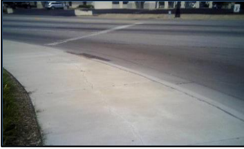
Corner 1 No Ramp (1z)
