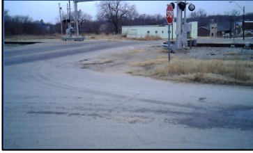
Corner 1 No Ramp (1z)
