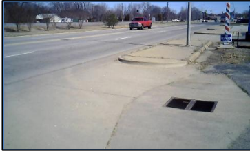
Corner 3 No Ramp (3z)
