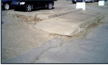
Corner 1 No Ramp (1z)
