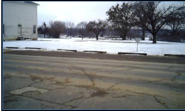
Corner 4 No Ramp (4z)
