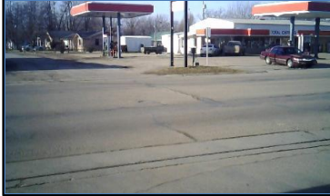
Corner 4 No Ramp (4z)
