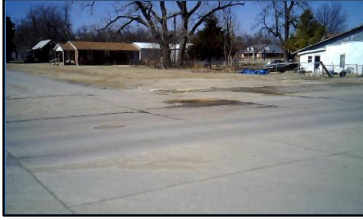
Corner 1 No Ramp (1z)
