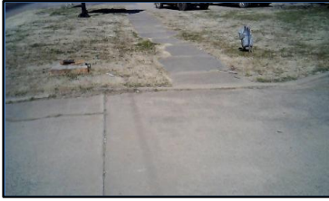
Corner 2 No Ramp (2z)
