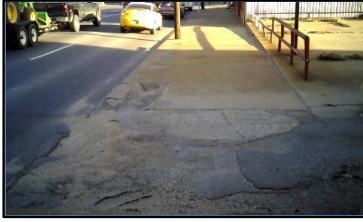
Corner 2 No Ramp (2z)
