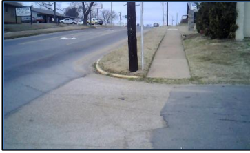
Corner 1 No Ramp (1z)
