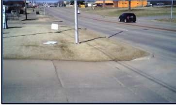
Corner 4 No Ramp (4z)
