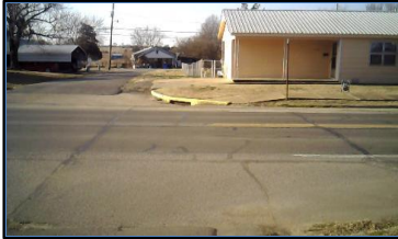
Corner 4 No Ramp (4z)
