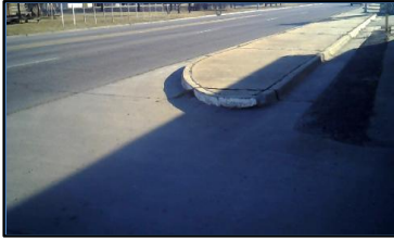
Corner 3 No Ramp (3z)
