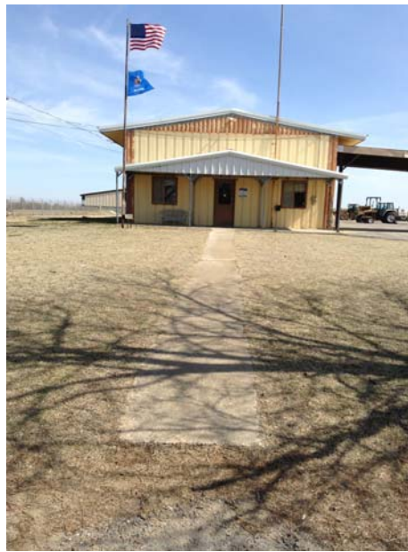
2. Accessible Route Violation 1
