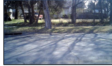
Corner 3 No Ramp (3z)
