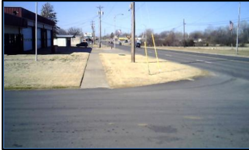
Corner 4 No Ramp (4z)
