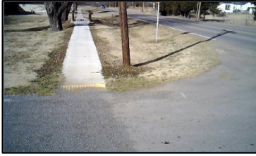
Corner 1 No Ramp (1z)
