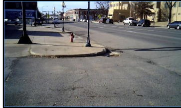
Corner 4 No Ramp (4z)
