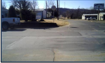
Corner 4 No Ramp (4z)
