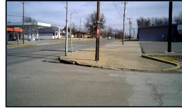
Corner 3 No Ramp (3z)
