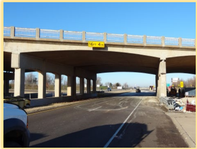
Figure 2: Substandard Vertical Clearance under I-40 at Anderson Road
