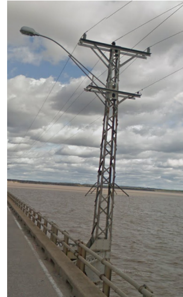
Luminaires on Bridge
