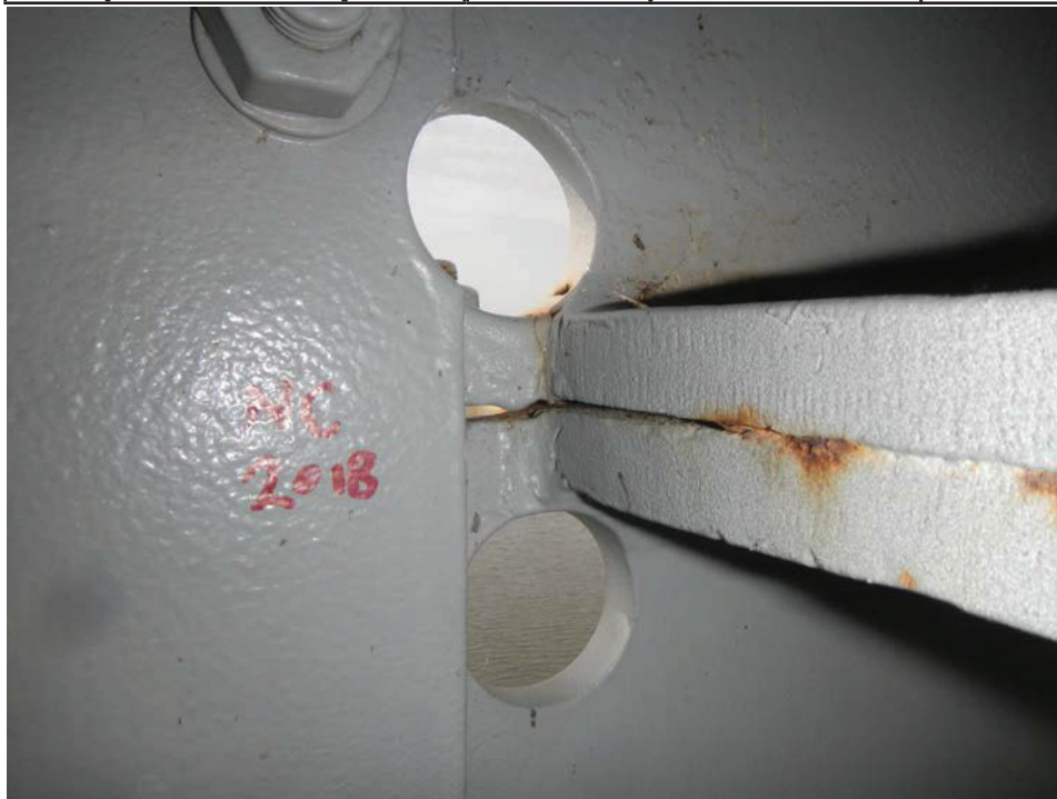
Photograph 8 - Looking southwest at girder 1, span 6 at the termination of the horizontal splice near floor beam 3. Note: 3/4-inch long crack arrested with drilled hole retrofits.
