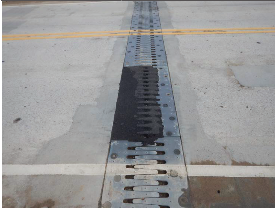
Photograph 5 - Looking north along the finger expansion joint at pier 4. Note: 5-foot section of the finger joint has been repaired with an asphalt patch.
