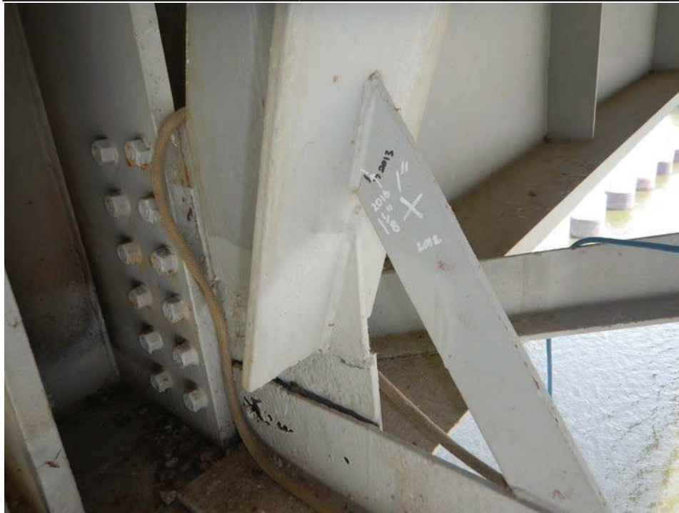
Photograph 21 - Looking northeast at the connection plate for floor beam 0, span 6 at girder 2 bottom flange. Note: 1/2-inch and 1 1/8-inch long cracks in welded repair plate.
