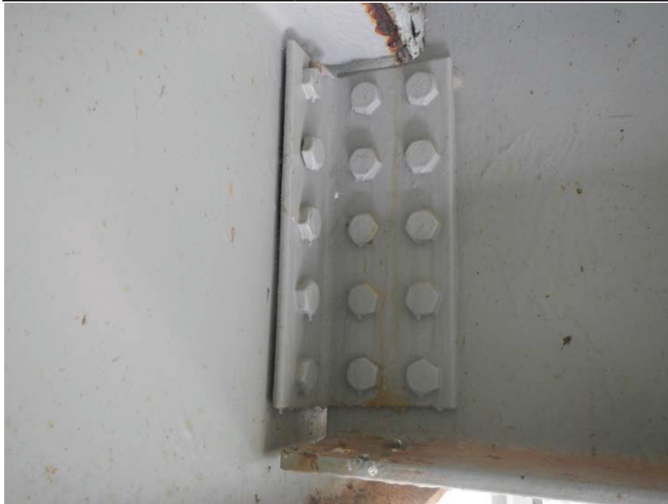
Photograph 18 - Looking northwest at the stringer 1 connection to floor beam 11 in span 6. Note: 5 loose bolts in connection angle to the floor beam web.
