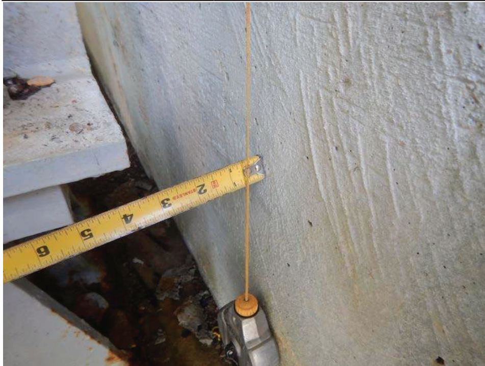
Photograph 24 - Looking north at the east abutment backwall at girder 1. Note: backwall is leaning 11/16 inch over 4 feet.
