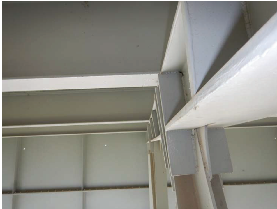
Photograph 19 - Looking south along floor beam 1, span 7. Note: gusset plate at stringer 3 is bent between the two diagonals up to 9/16 inches. The floor beam bottom flange is twisted and rolling to the east up to 8 degrees near midspan.
