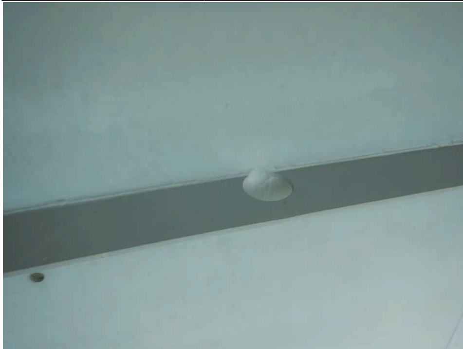
Photograph 12 - Looking north at girder 1, span 6 near floor beam 6. Note: drilled retrofit in upper horizontal stiffener.
