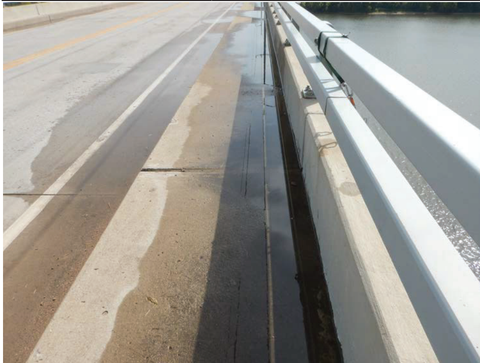
Photograph 3 - Looking east along the south bridge rail at floor beam 6, span 6. Note: ponding water on the sidewalk in span 6.
