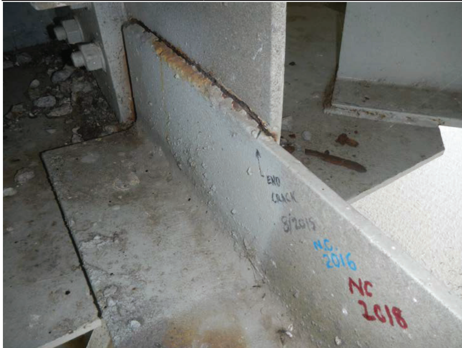
Photograph 20 - Looking northeast at the connection plate for floor beam 0, span 6 at the girder 2 bottom flange. Note: the horizontal weld has cracked full length.
