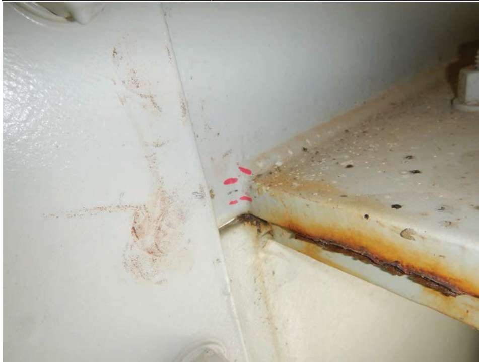
Photograph 7 - Looking northeast at girder 2, span 5 at the termination of the horizontal splice east of floor beam 5. Note: new 1/2-inch long paint crack adjacent to the previously noted 3/8-inch long paint crack.
