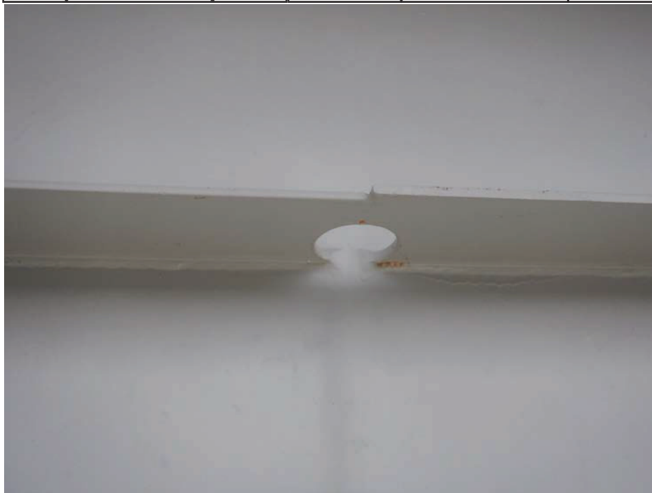
Photograph 14 - Looking north at girder 1, span 6 near floor beam 9. Note: drilled retrofit in upper horizontal stiffener.
