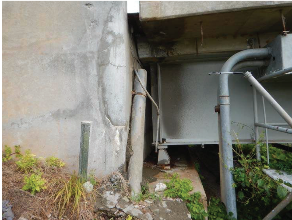
Photograph 23 - Looking north at the west abutment. Note: backwall has rotated east 1 1/8 inches over 4 feet.
