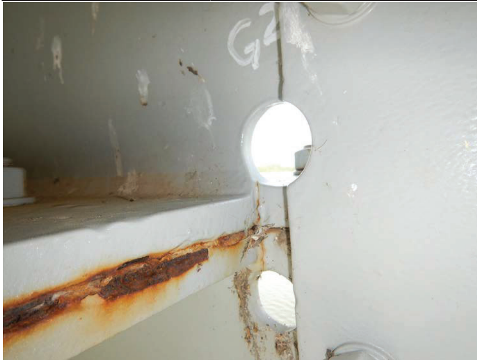
Photograph 10 - Looking northwest girder 2, span 7 at the termination of the horizontal stiffener near floor beam 4. Note: two vertical cracks arrested with drilled hole retrofits. No change from the 2017 inspection.
