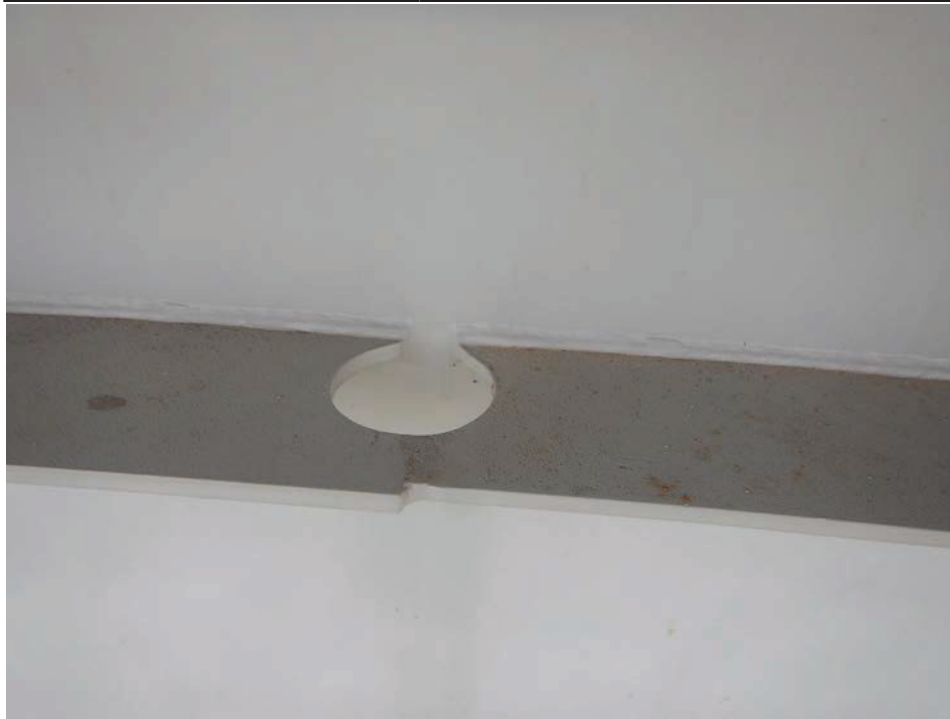
Photograph 15 - Looking south at girder 2, span 6 near floor beam 9. Note: drilled retrofit in upper horizontal stiffener.
