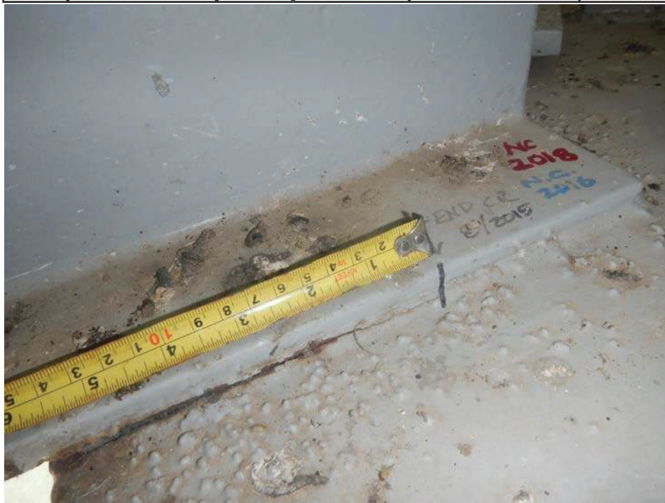
Photograph 22 - Looking west at the lower lateral bracing connection to the gusset plate at girder 2, east face of floor beam 12 in span 6. Note: 5 5/8-inch long crack in the weld between the bottom angle and the bracing gusset plate, no change since last inspection.
