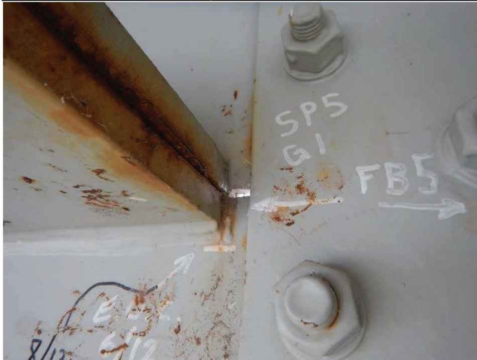
Photograph 6 - Looking southeast at girder 1, span 5 at the termination of the horizontal splice near floor beam 5. Note: no change to previously noted crack.
