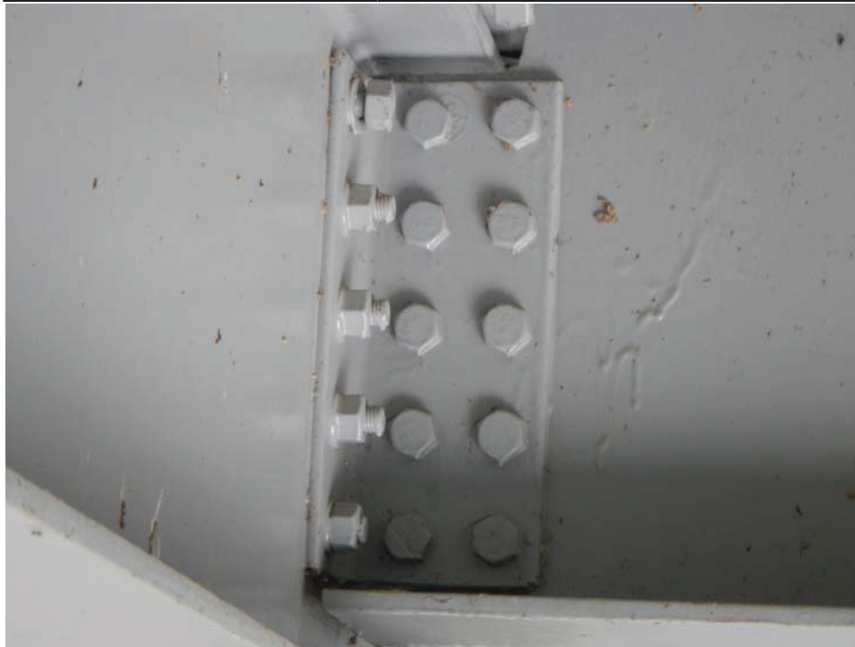
Photograph 17 - Looking north at the stringer 2 connection to floor beam 3 in span 6. Note: 1 loose bolt in connection to the floor beam.
