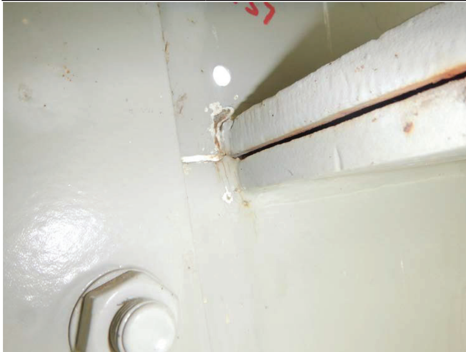
Photograph 9 - Looking southwest at girder 1, span 7 at the termination of the horizontal splice near floor beam 4. Note: paint cracks up to 1 inch long at the top plate and 1 1/8 inches long at the bottom plate. No change from 2017 inspection.
