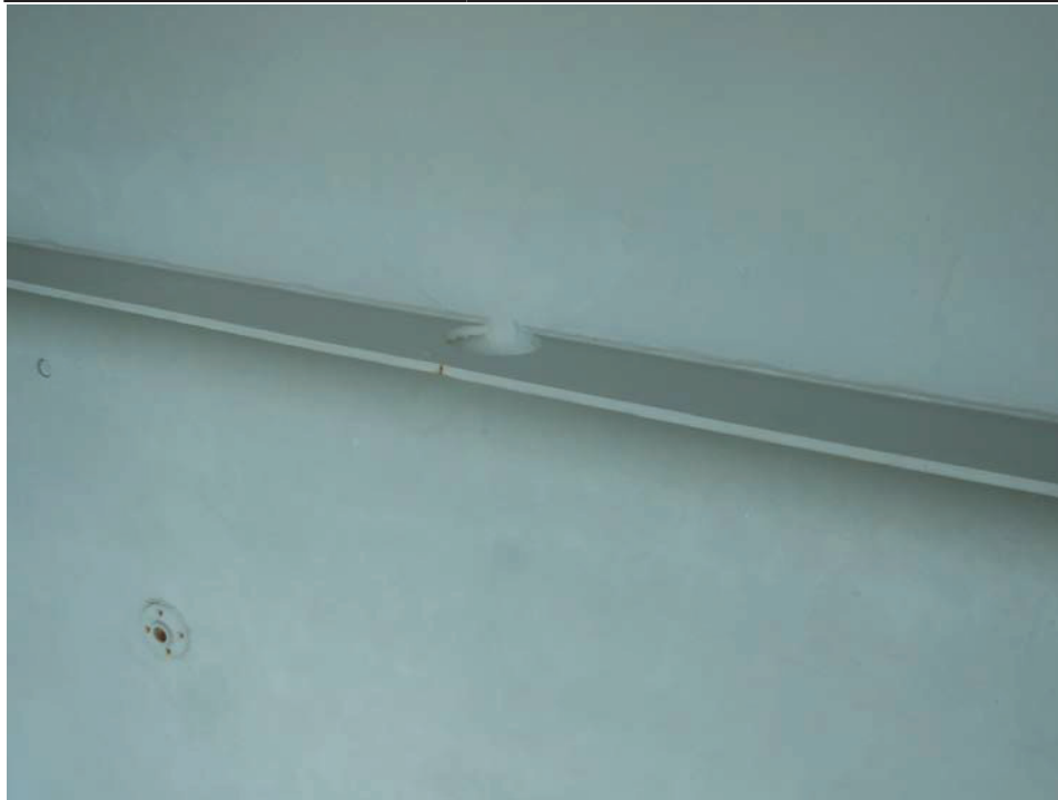
Photograph 13 - Looking north at girder 1, span 6 near floor beam 7. Note: drilled retrofit in upper horizontal stiffener.
