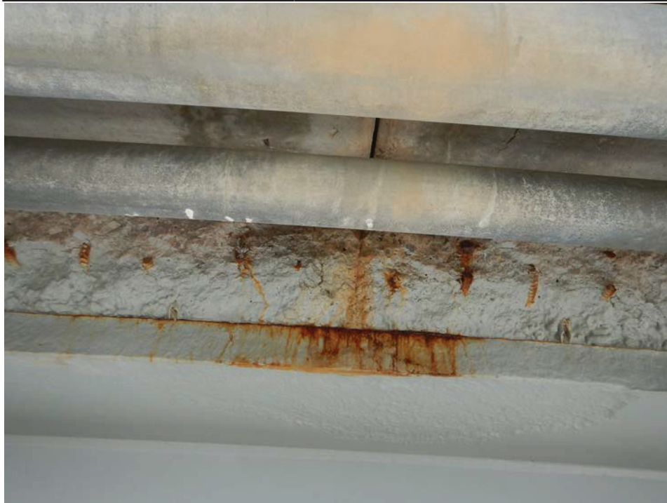
Photograph 4 - Looking north at the underside of the south overhang at floor beam 6, span 6. Note: spalling of the deck and corrosion of girder 1 due to deck drainage ponding on the sidewalk.
