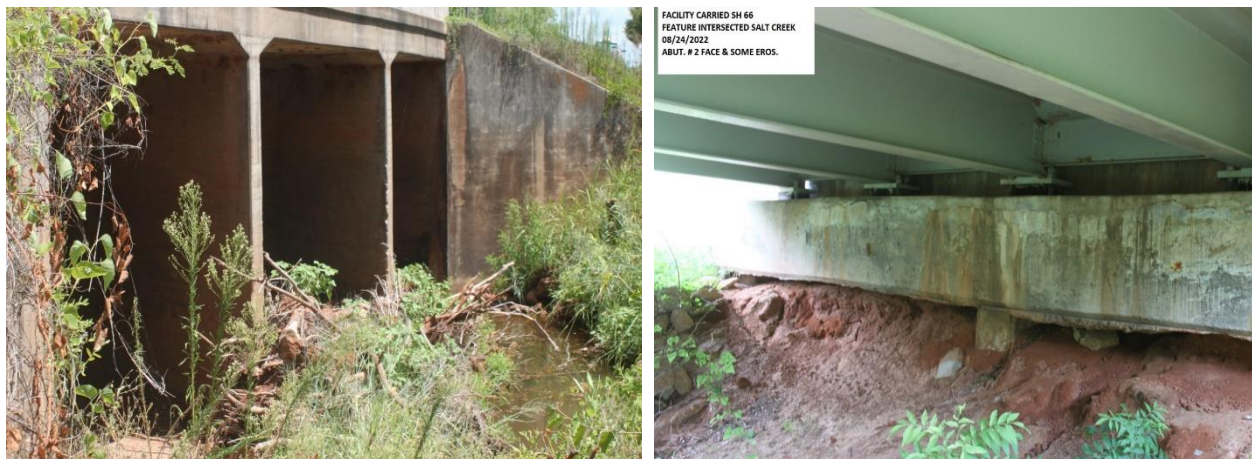
Figure 13: Deterioration of Structures Caused by Stormwater Runoff
