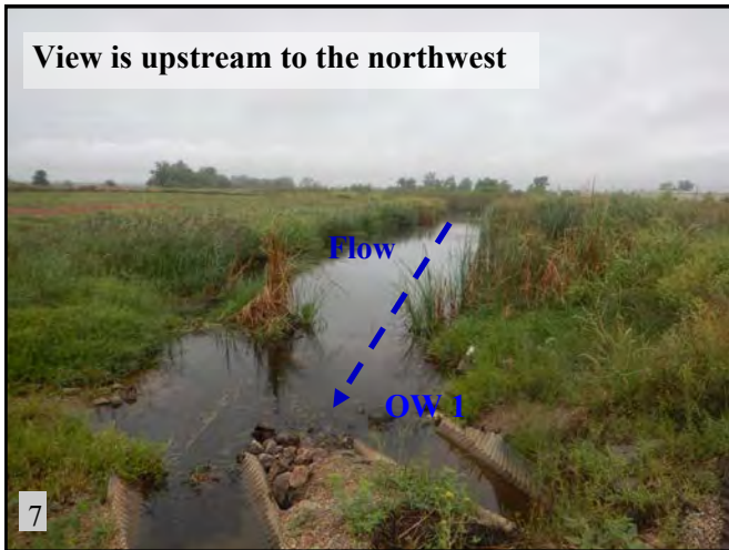
▲(PS 3): View of OW 1 and double CGMP culvert under S. Harvey Ave.
