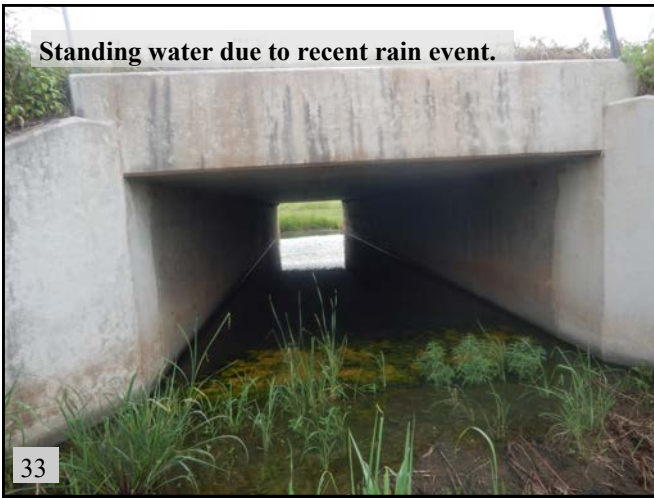
▲ (PS 14): View of RCB under NW 12th Ave. with cliff swallow nests. View is to the east.
