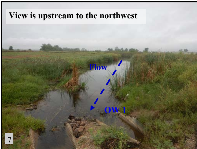
▲(PS 3): View of OW 1 and double CGMP culvert under S. Harvey Ave.
