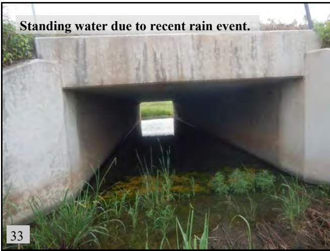
▲ (PS 14): View of RCB under NW 12th Ave. with cliff swallow nests. View is to the east.
