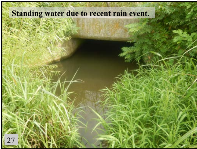
▲ (PS 11): View of RCB under SH-9 and near Wetland 4. View is to the south.
