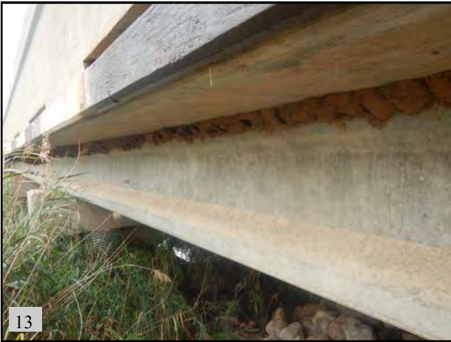
▲ (PS 5): Past use by cliff swallows under NBI 27477. View is to the northeast.
