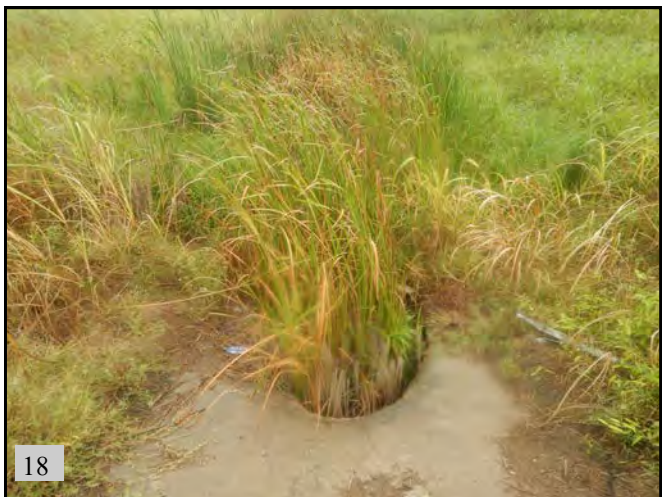
▲ (PS 7): View of Wetland 3 and culvert under S. Harvey Ave. View is to the east.
