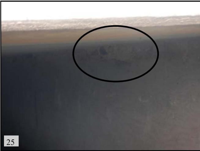
▲ (PS 10): View of the RCB under S. Harvey Ave. and cliff swallow nest (circled). View is to the east.
