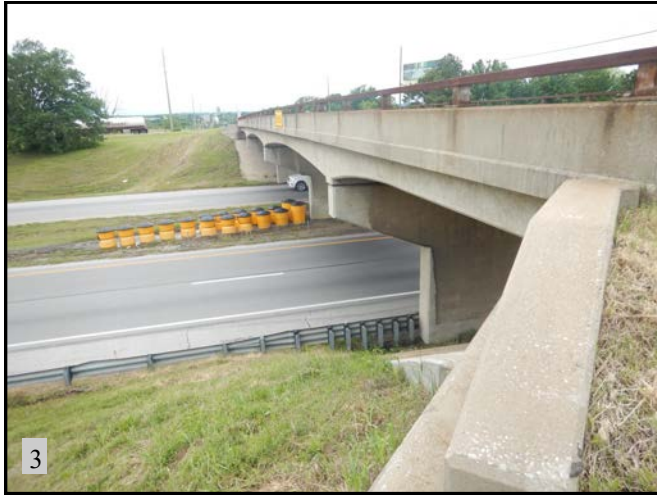
▲ (PS 2): View of NBI 16564. Bridge was not fully inspected due to height and safety. View is to the west.
