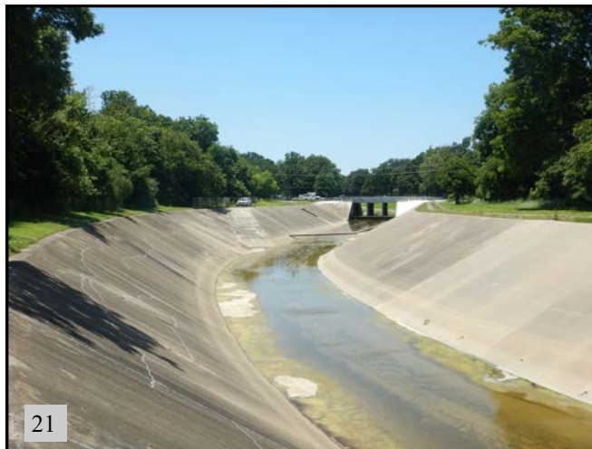
▲(PS 7): Concrete lined Cherry Creek (OW 5). View is upstream to the west.
