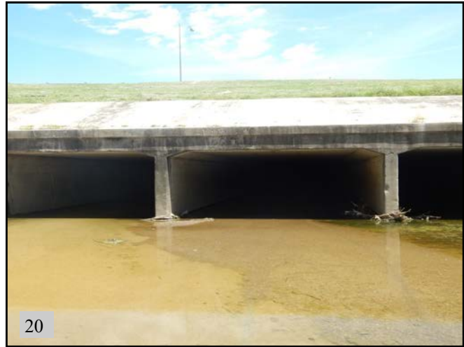
▲(PS 10): Triple cell RCB over Cherry Creek (OW 5). View is downstream to the east.
