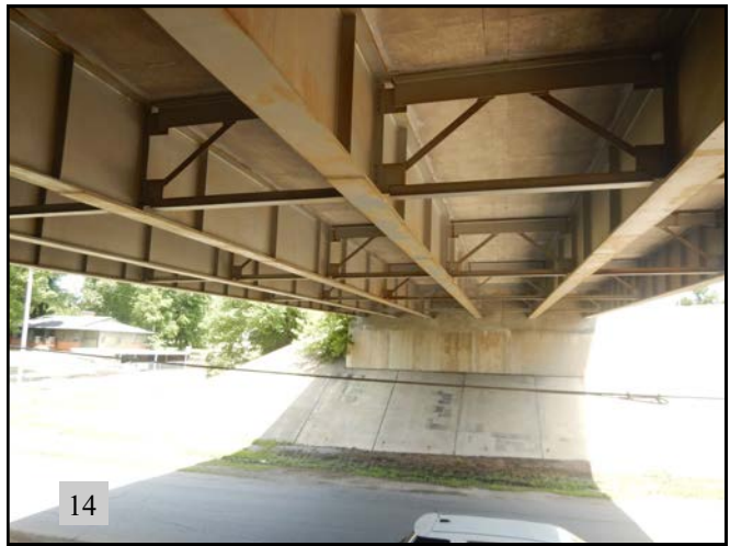
▲(PS 7): View under NBI 18268 over W. 49th St. View is to the south.
