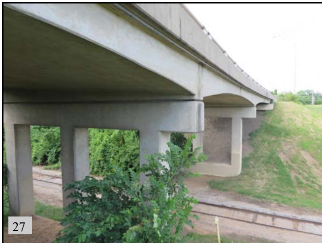
▲ (PS 16): View of NBI 15755. Bridge could not be fully inspected due to height. View is to the west.
