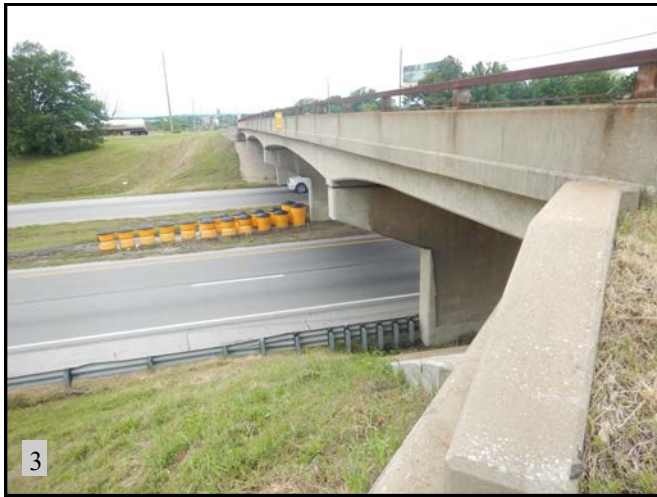
▲ (PS 2): View of NBI 16564. Bridge was not fully inspected due to height and safety. View is to the west.
