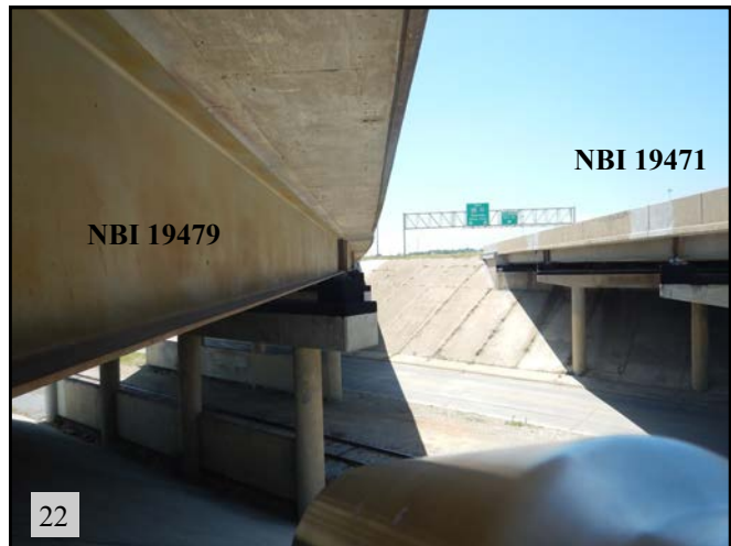
▲(PS 11): Inspecting bridge for bat and/or migratory bird use. View is to the west.
