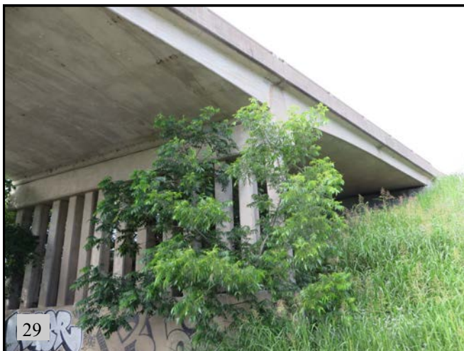
▲ (PS 18): View of NBI 15763. Bridge could not be fully inspected due to height. View is to the southeast.
