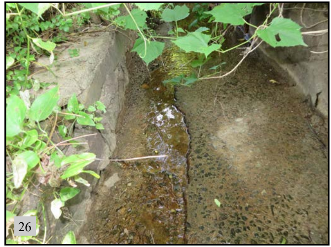
▲ (PS 15): View of the concrete lined channel and stone banks of OW 7. View is downstream to the south.
