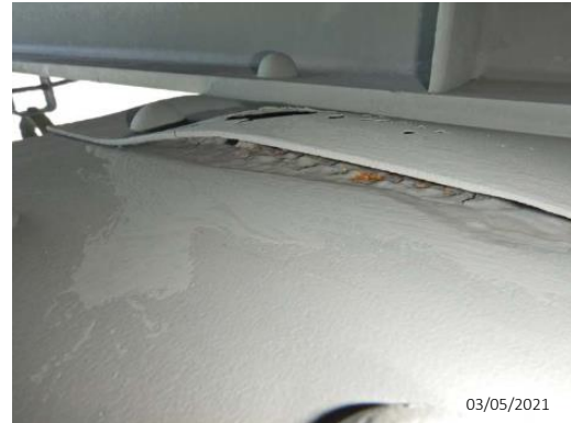
Figure 25: Inspection Photo: Primary Girder Pitting
