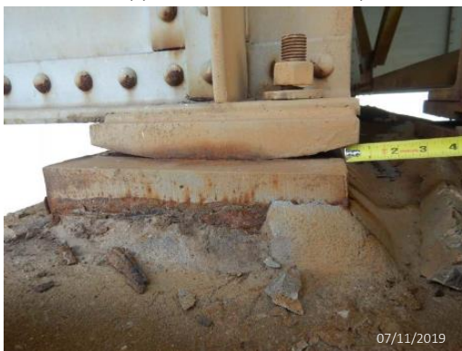
Figure 29: Inspection Photo: Shifted Rocker Bearing
