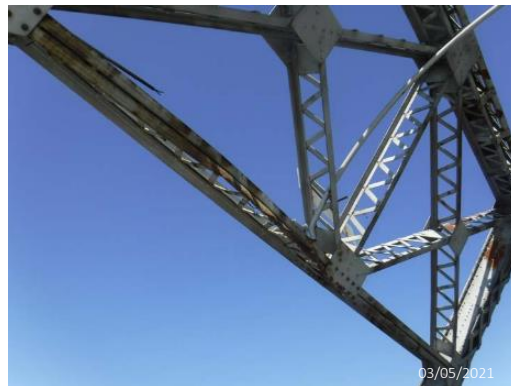
Figure 36: Inspection Photo: Damaged Portal Bracing
