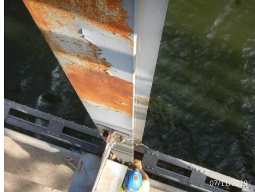
Figure 34: Inspection Photo: Truss Vertical Member Misalignment
