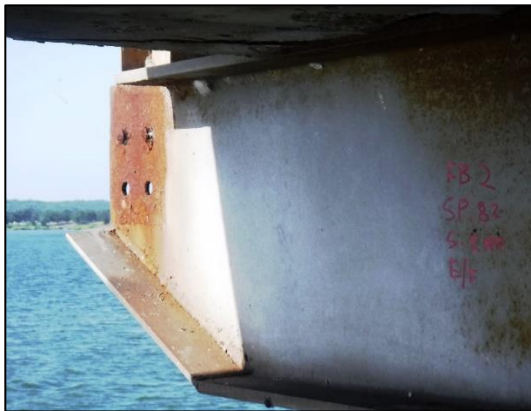
Figure 59: Missing Rail Connection
