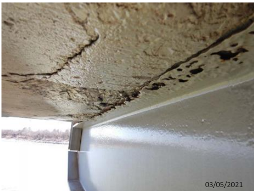
Figure 22: Inspection Photo: Floor Beam Section Loss & Knife Edging in Top Flange
