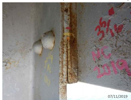
Figure 33: Inspection Photo: Crack in Fill Plate Adjacent to Vertical Inside Upper Panel Point
