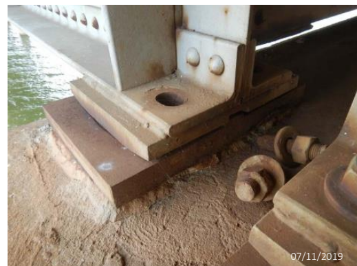
Figure 30: Inspection Photo: Sheared Bolts at Bearing
