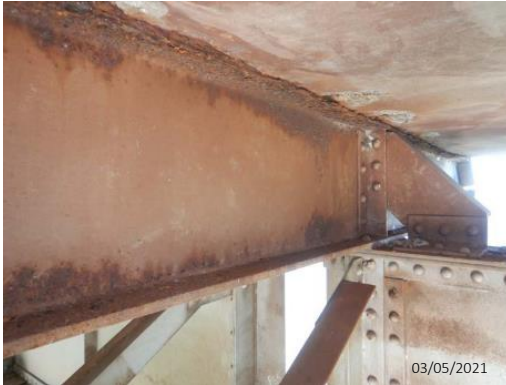
Figure 27: Inspection Photo: Floor Beam Section Loss & Corrosion
