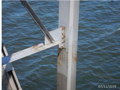
Figure 35: Inspection Photo: Relocated Sway Bracing Connection
