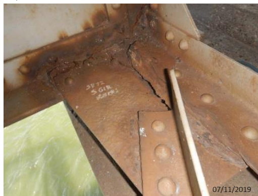
Figure 26: Inspection Photo: Bracing Corrosion
