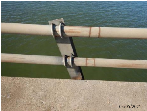
Figure 20: Inspection Photo: Failed Rail Post
