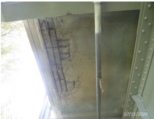
Figure 18: Inspection Photo: Deck Soffit Spall
