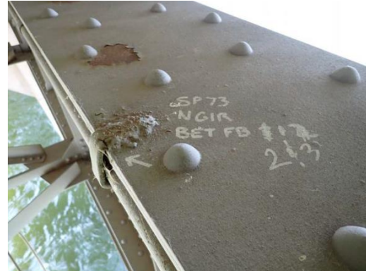
Figure 28: Inspection Photo: Cracks in Connected Bracket Welds
