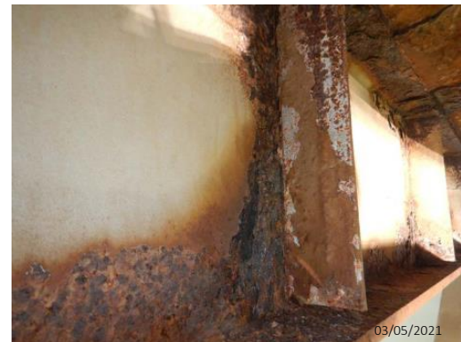
Figure 23: Inspection Photo: Floor Beam Section Loss & Corrosion in Web
