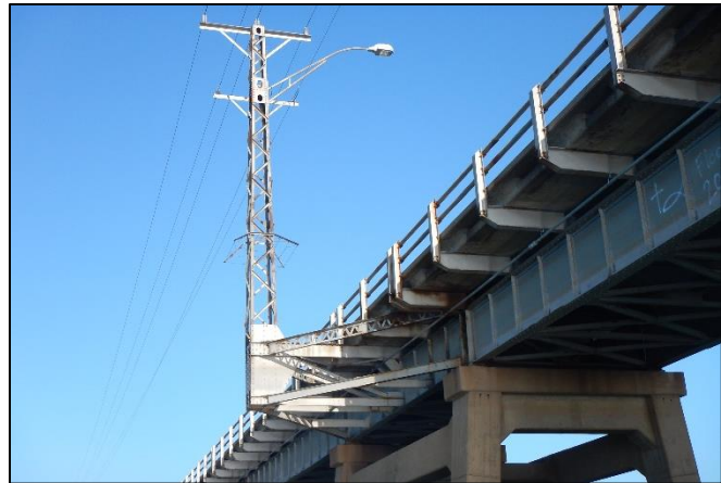
Photo 20: Typical Bridge Lighting
