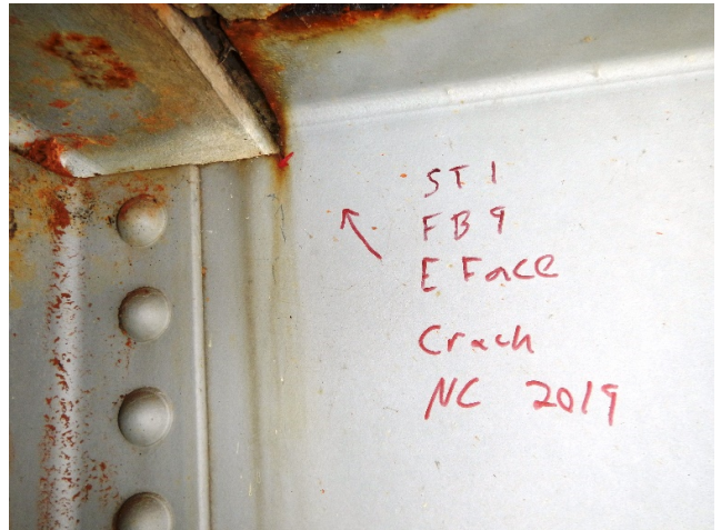
Photo 14: Cracking at Re-entrant Corners of Stringers
