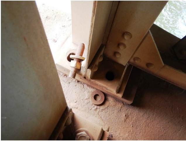
Photo 17: Broken Anchor Bolts
