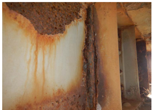
Photo 16: Built-Up Primary Girders with Section Loss of Webs Near Angle Stiffeners
