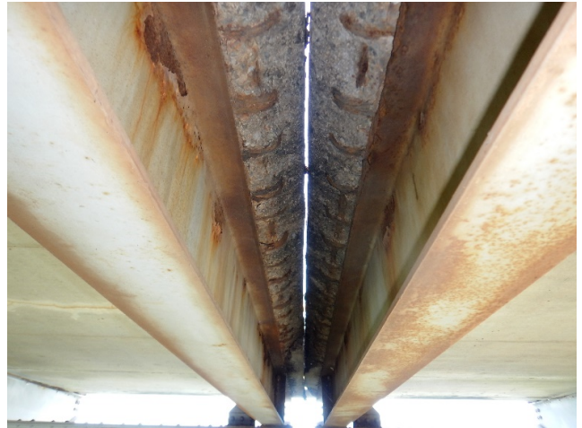
Photo 12: Soffit at Joints with Partial Depth Spalling
