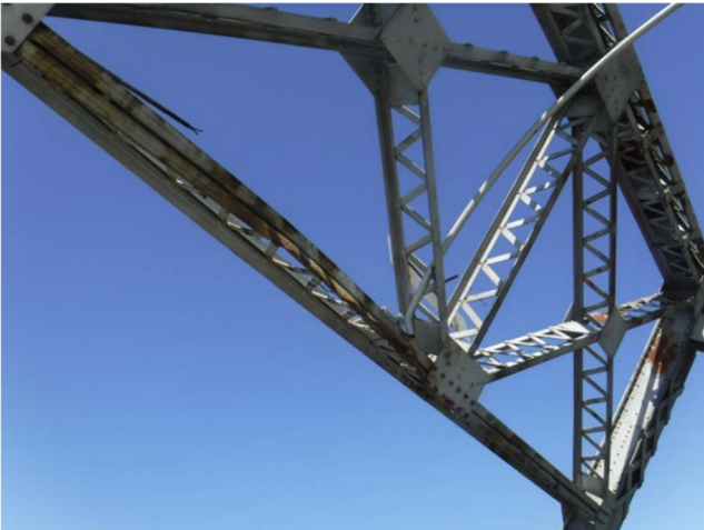
Photo 7: Portal Strut Vehicular Collision Damage
