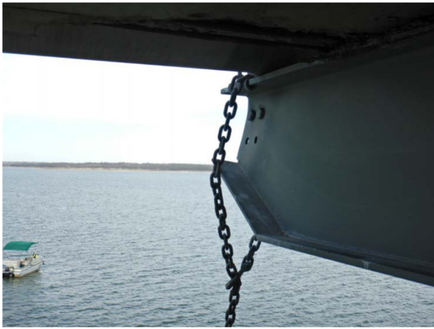
Photo 10: Deflected Floor Beam Due to Vehicular Collision to Traffic Rail
