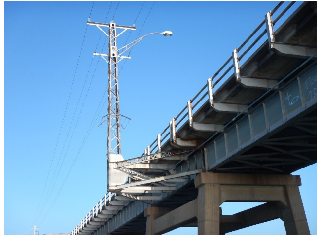
Photo 20: Typical Utility Tower
