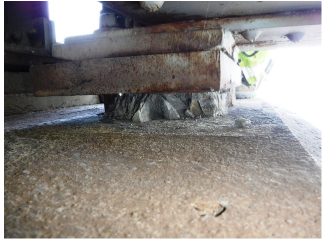
Photo 18: Loss of Grout Pad Beneath Primary Girders
