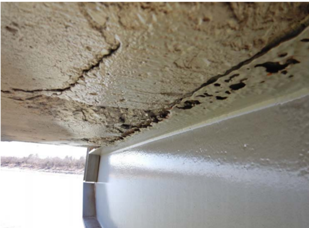
Photo 13: Floor Beam Substantial Section Loss of Top Flange
