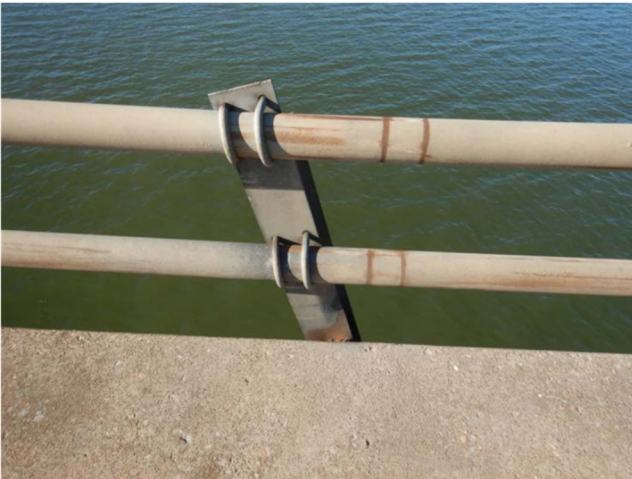
Photo 6: Traffic Rail Damage Due to Vehicular Collision
