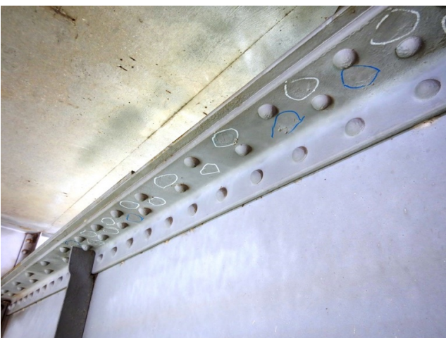
Photo 15: Built-Up Primary Girders with Plug Welds in Rivet Holes (Fatigue Concern)
