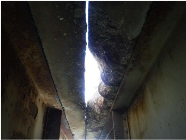
Photo 11: Soffit at Joints with Full Depth Spalling
