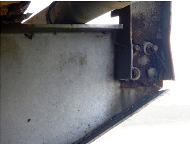
Photo 9: Failed Traffic Rail Connection to Floor Beam
