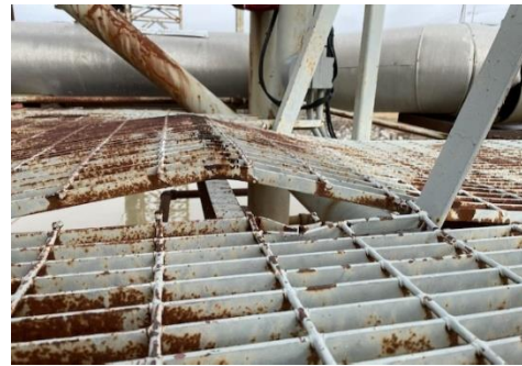
Tulsa Port of Catoosa – Platform Critical Failure
