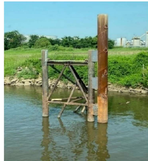
Figure 7. Existing dolphins at Port Muskogee (pictured above) and TPOC will be replaced with safer, more efficient monopile and dolphin mooring infrastructure.
