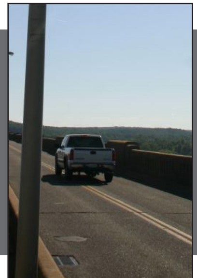
Truck Driving over Center Line on Narrow Bridge
