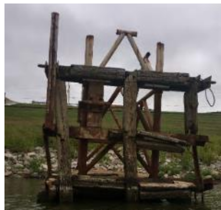
Tower dolphin structure in disrepair at Tulsa Port of Catoosa
