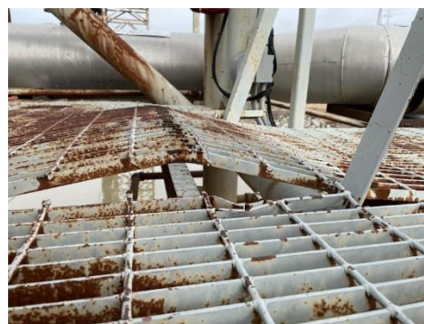
Tulsa Port of Catoosa – Platform Critical Failure
