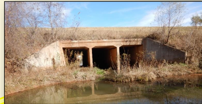
Hog Creek – 3 Cell Reinforced Concrete Box
