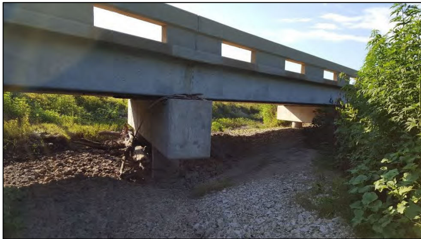
Photo 11 – Bridge at Whiskey Creek Road with unnamed tributary in the central project area, facing west.
