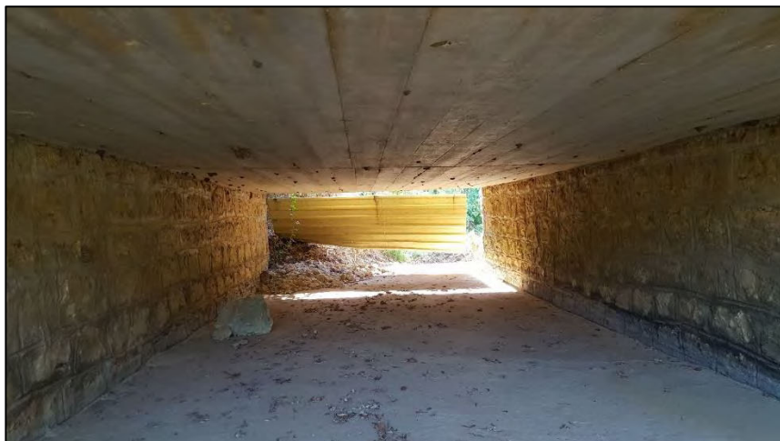
Photo 9 – Within the study footprint, bridges and culverts (such as this one) were inspected for swallows nests.
