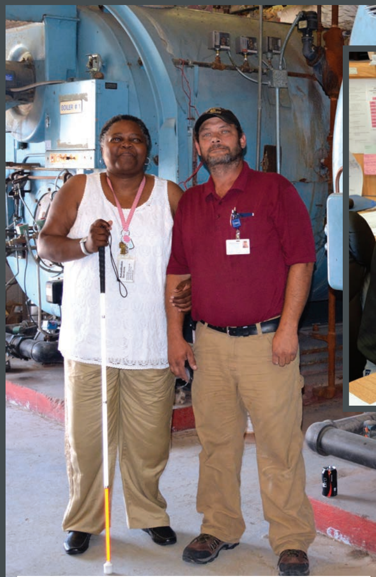
Above: Gayle Lee and Alex Pippins at his job near the chillers he works on at McAlester Regional Health Center. Right: David Parish and Pippins go over paperwork and work orders.
