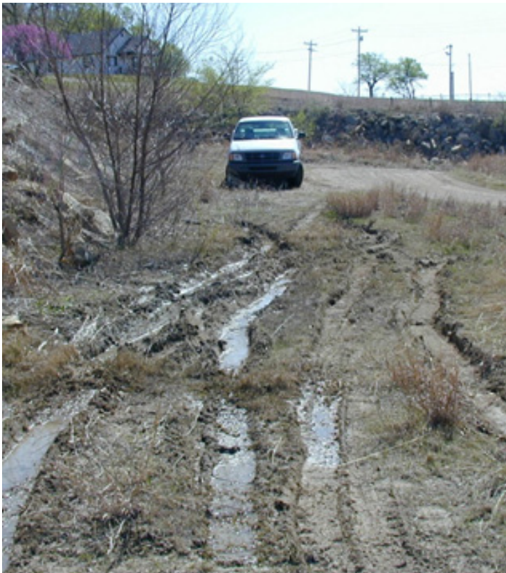
FIGURE 5.5. AREA OF SEEPAGE NEAR TOE OF DAM.
