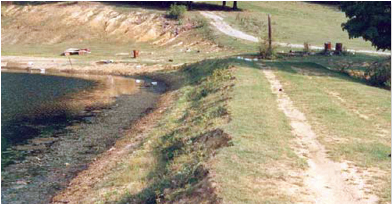
FIGURE 7.2. BENCHING DUE TO WAVE EROSION OF UPSTREAM SLOPE OF DAM.
