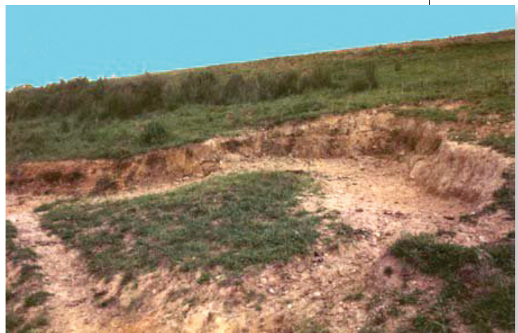
FIGURE 7.1. EROSION OF EMBANKMENT WITH POOR COVER
