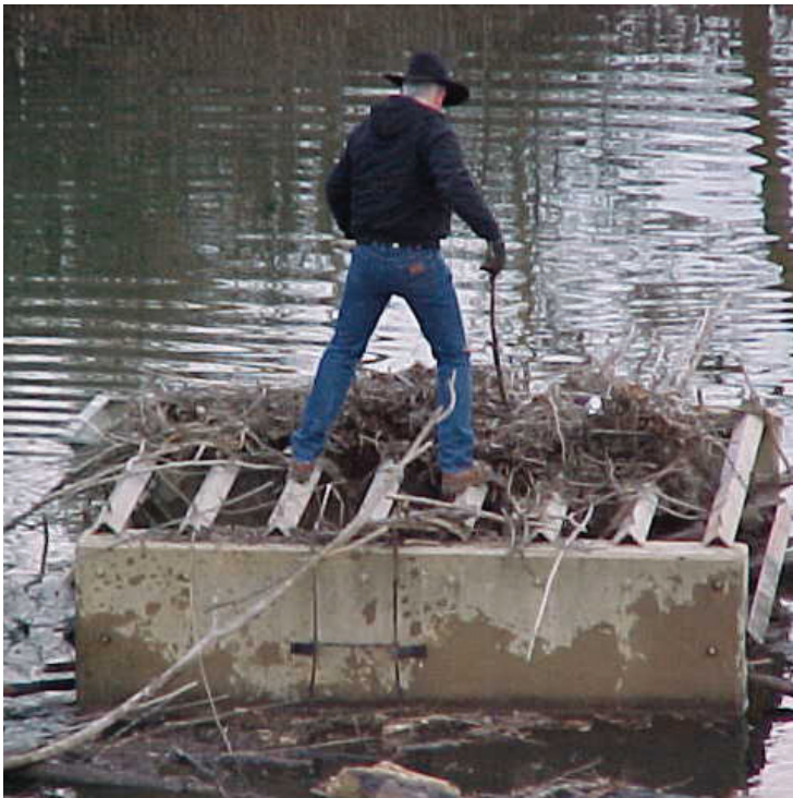
FIGURE 5.7. KEEPING TRASH RACKS FREE OF DEBRIS REDUCES THE CHANCE OF OVERTOPPING THE DAM.
