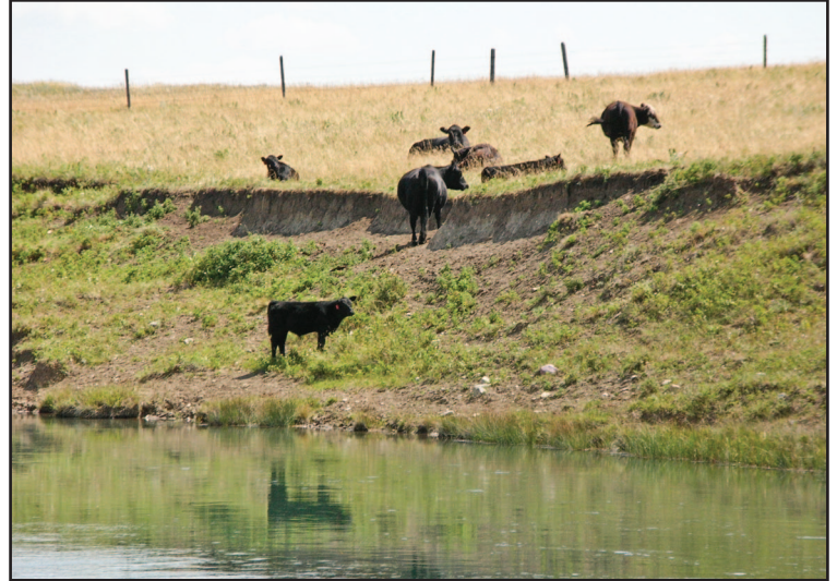
Figure 18—Livestock paths on dam faces can lead to dam erosion.
