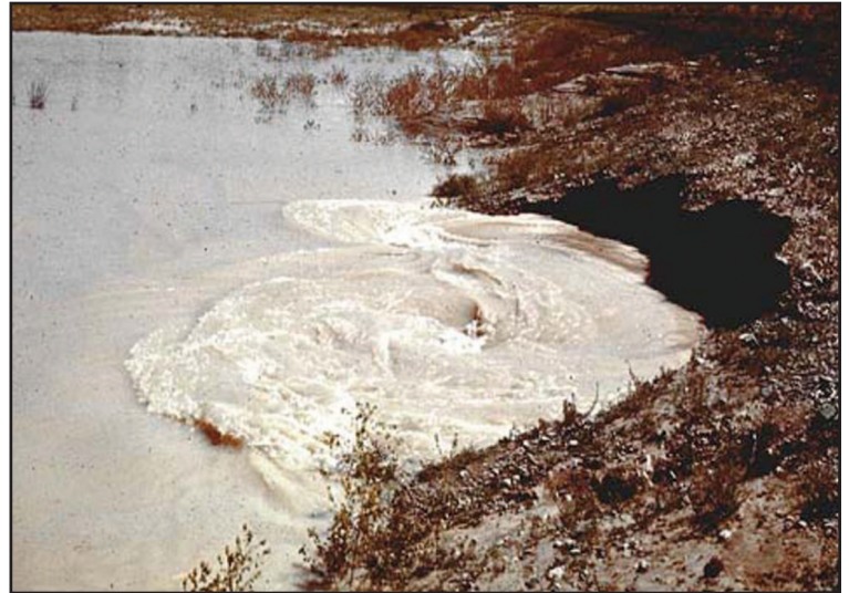
Figure 6—Whirlpool action is an indication of advanced piping.
