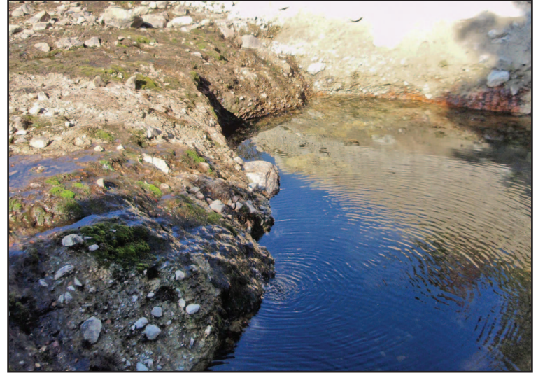
Figure 40—Erosion of the spillway channel may lead to slumps or slides of the spillway sides.
