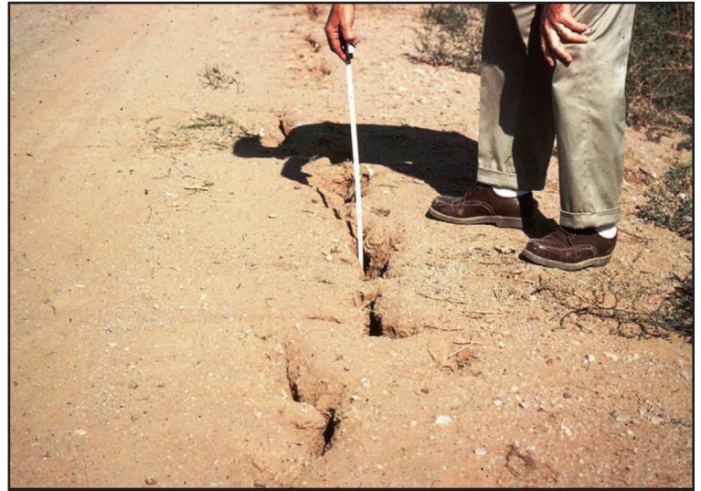
Figure 22—Longitudinal cracks can be an indication of dam instability.
