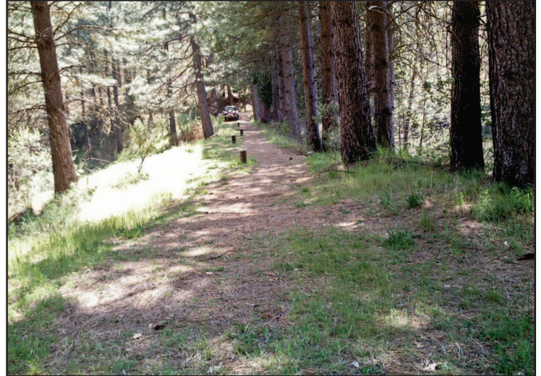
Figure 14—Trees growing on the crest and the faces of a dam.
