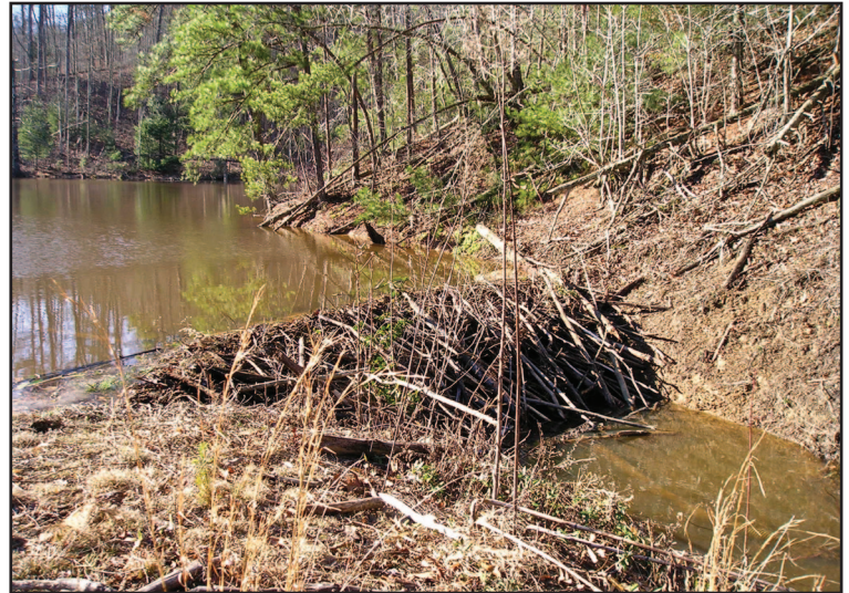
Figure 38—A blocked spillway channel may cause overtopping of the dam.
