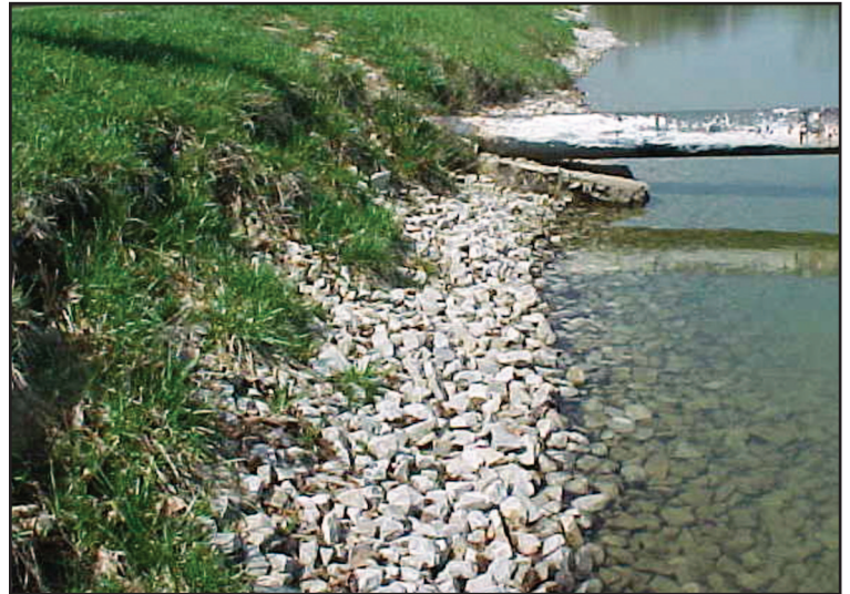
Figure 10—Wave erosion on the unprotected face of a dam.
