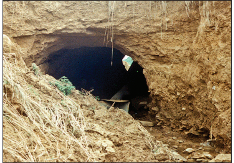
Figure 32—Piping of water alongside an outlet pipe.
