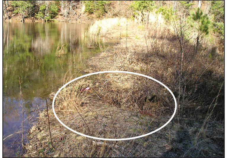
Figure 24—Low areas in the crest of a dam reduce the freeboard.
