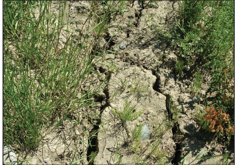
Figure 20—Transverse cracks can be an indication of dam instability.
