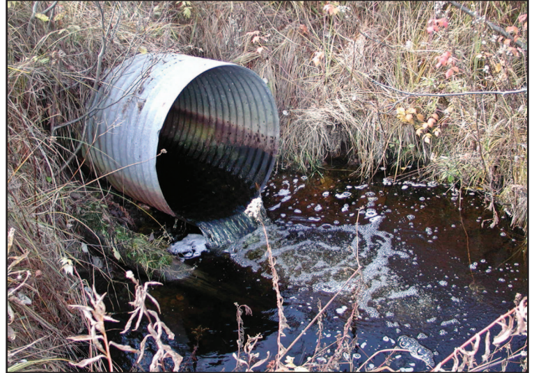
Figure 36—A scour hole at an outlet erodes the toe of the slope.
