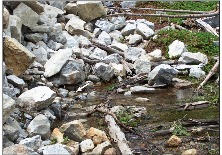
Figure 26—Excessive water piping through the dam at the toe of the embankment.
