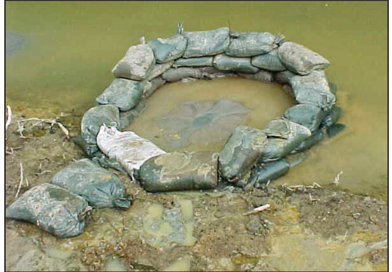
Figure 28— Sandbags surrounding a boil on the downstream side of the dam.
