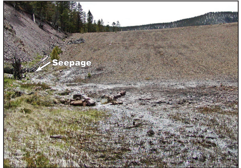
Figure 30—Seepage at the abutment contact (groin) can lead to dam failure.
