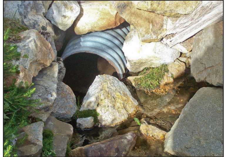
Figure 34—Rock failure around an outlet pipe.
